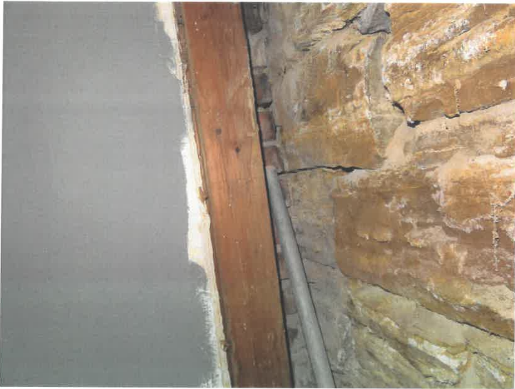
Photo 41 Building No. 20 – TNT Smoke House (366 Broadway St) Partial View of Filled-In Coal Chute w/ Brick on West Half of Building
