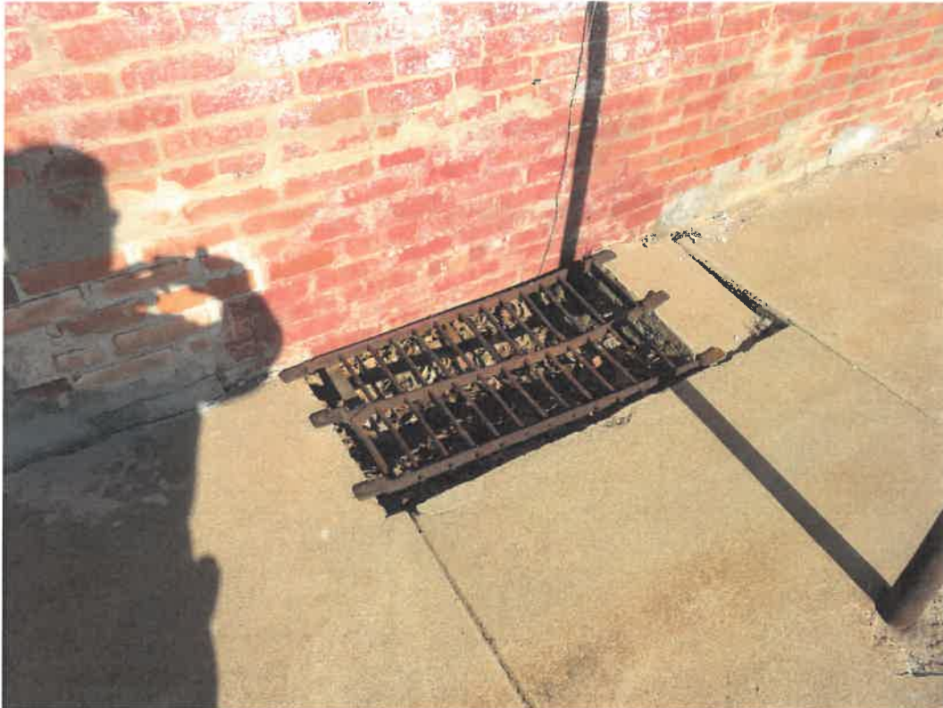
Photo 113 Building No. 45 – Hair by Luann (195 S 3rd St) Open Vent in Sidewalk on South Face of Building
