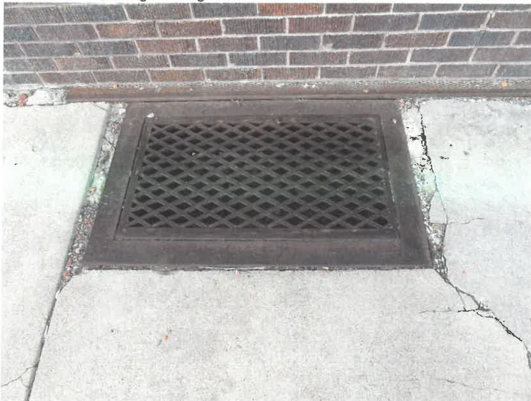
Photo 52 Building No. 23 – Steve Young Building (334 Broadway St) Open Coal Chute in Sidewalk
