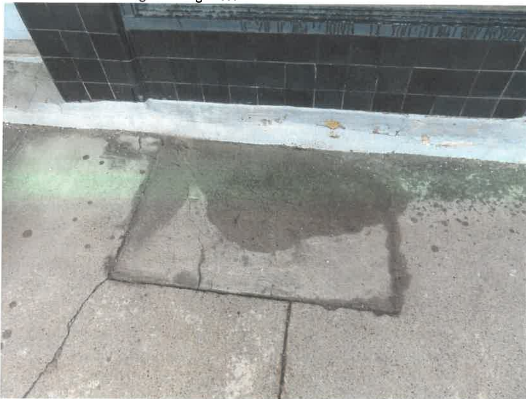
Photo 74 Building No. 33 – Tecumseh Chieftain (117 S 3rd St) Concrete Filled-In Coal Chute in Sidewalk
