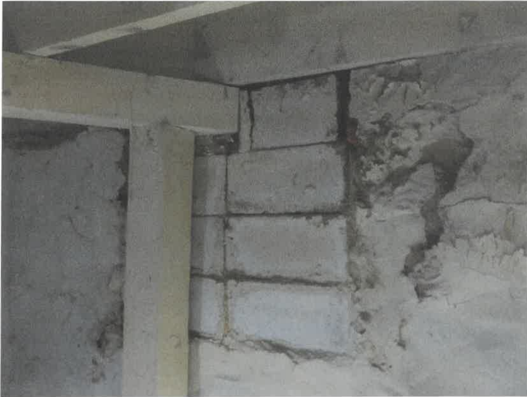
Photo 53 Building No. 23 – Steve Young Building (334 Broadway St) CMU Filled-In Coal Chute in Basement
