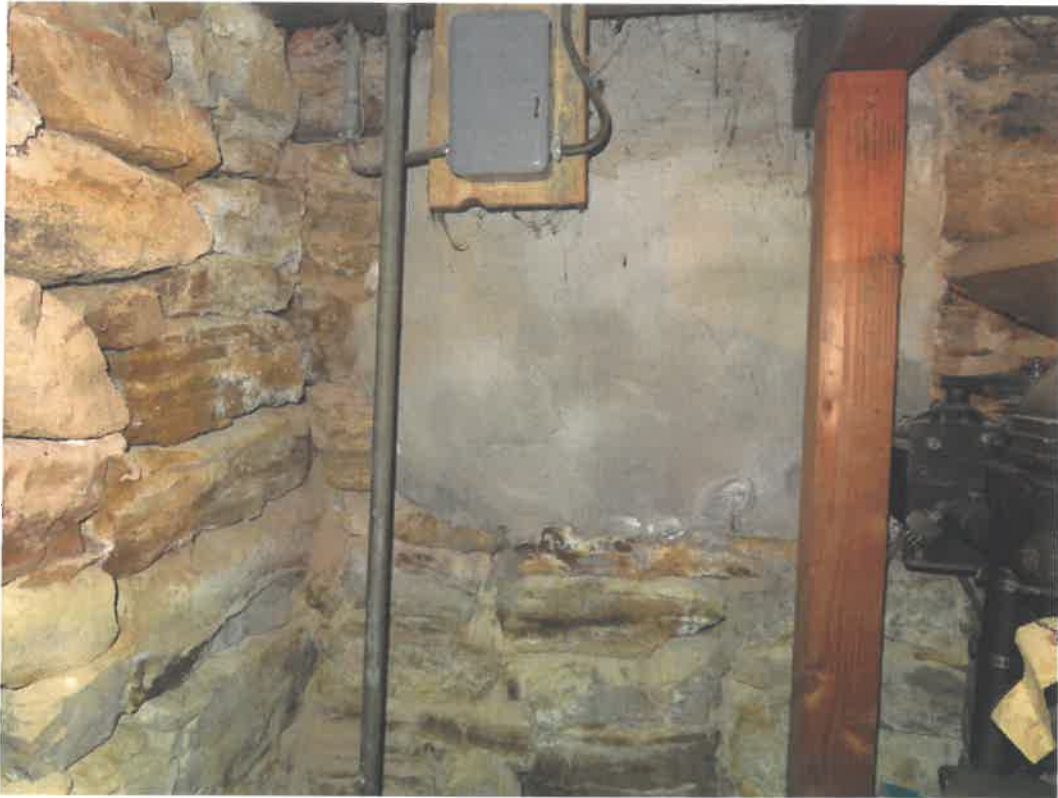
Photo 43 Building No. 21 – D.A. Wolken & Sons (362 Broadway St) Concrete Filled-In Coal Chute on East End of Building
