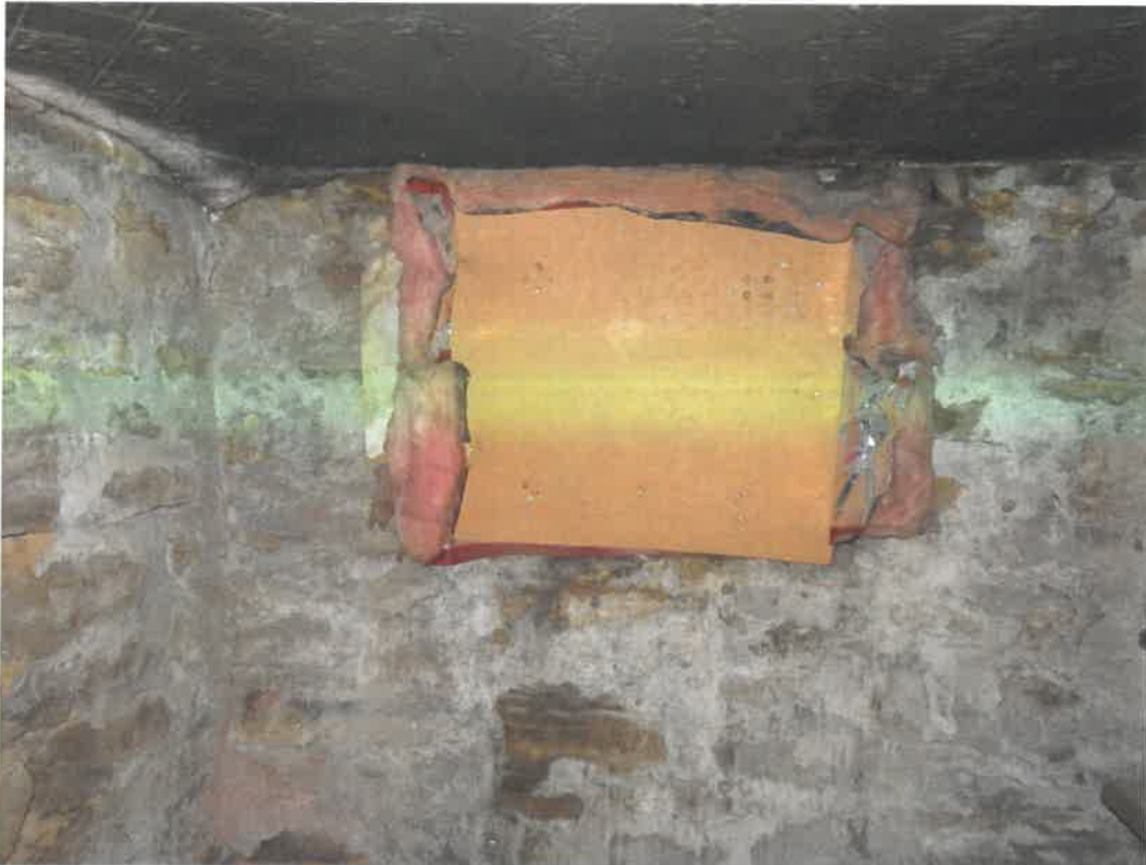
Photo 102 Building No. 42 – Morrissey, Morrissey & Dalluge (177 S 3rd St) Plywood/Insulation Filled-In Coal Chute in Basement
