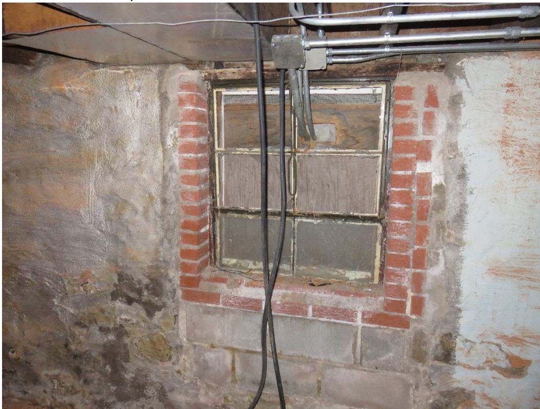
Photo 64 Building No. 26 – American National Bank (306/310 Broadway St) Partially Brick Filled-In Window at North End of West Wall in Basement
