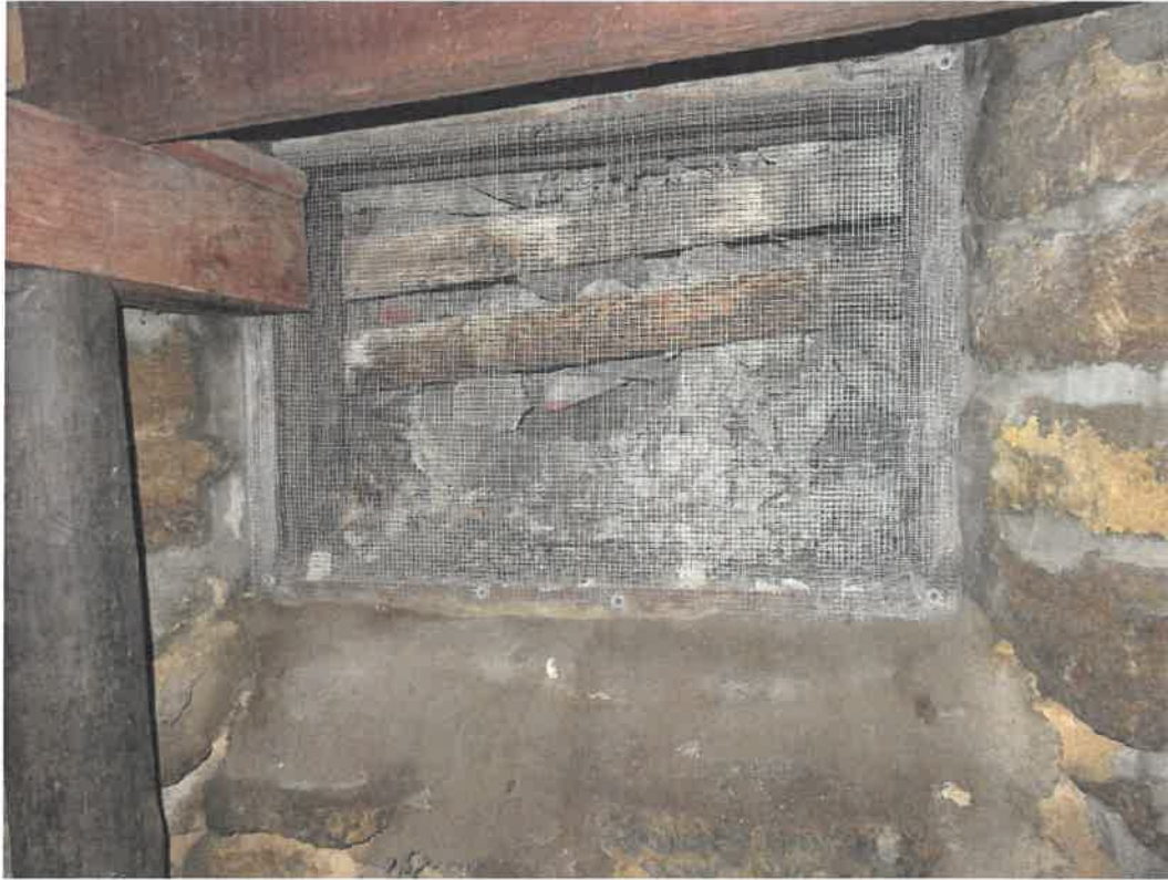
Photo 93 Building No. 39 – Remedy (171 S 3rd St) Rubble Filled-In Coal Chute in Basement
