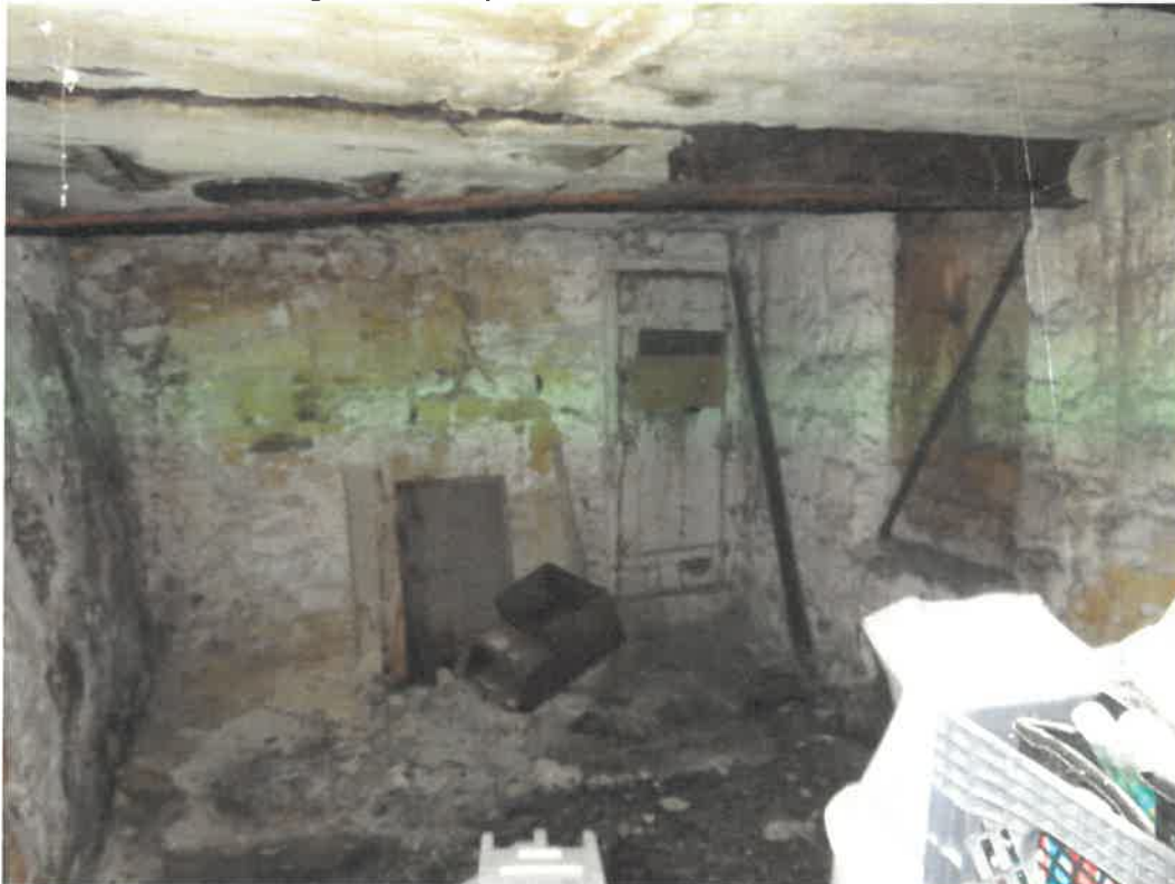
Photo 34 Building No. 17 – Nester & Mercure Attorneys (398 Broadway St) Looking South at Typical Deterioration in Vault 2 with Window on Right
