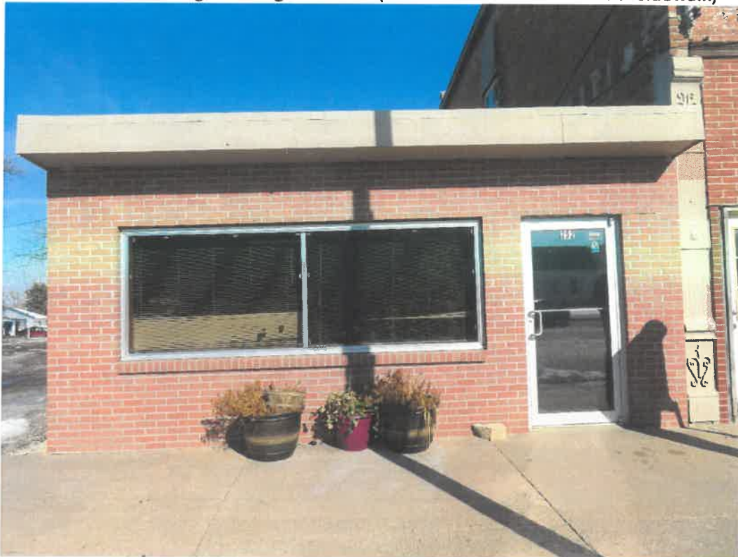
Photo 126 Building No. 49 – Gartner Transportation (252 Clay St) Frontage Looking North (Note: Vault Discovered Under Sidewalk)
