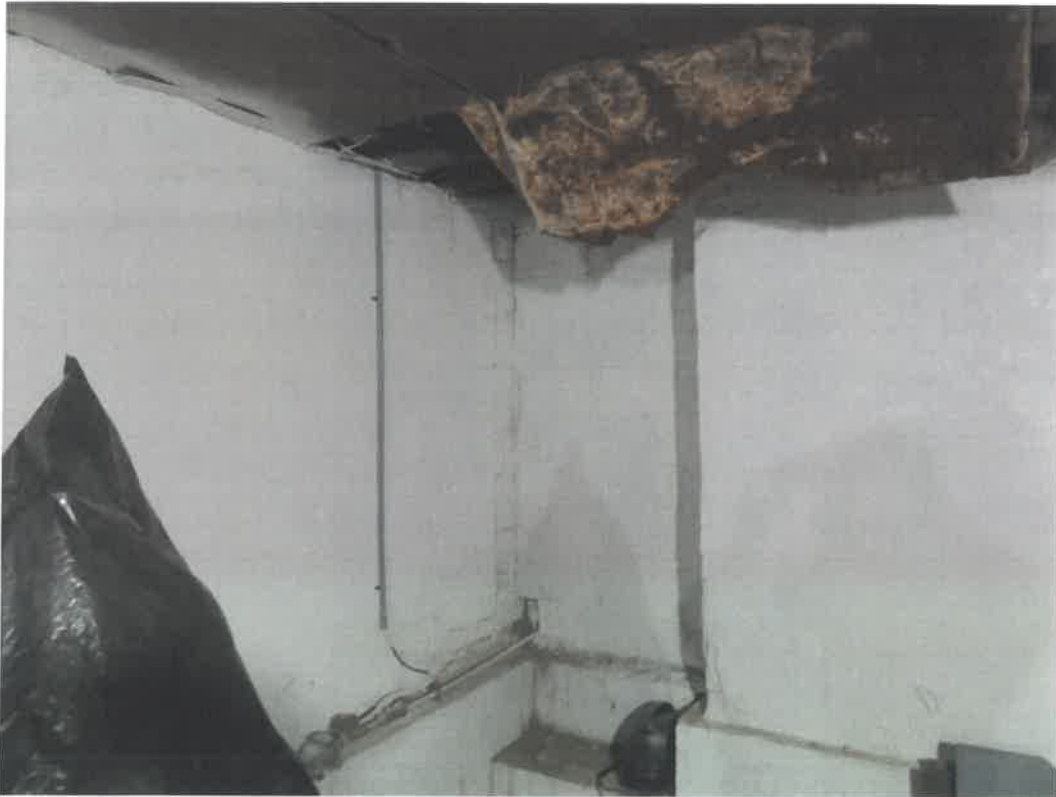
Photo 127 Building No. 49 – Gartner Transportation (252 Clay St) CMU Filled-In Door in Basement to Vault Under Sidewalk
