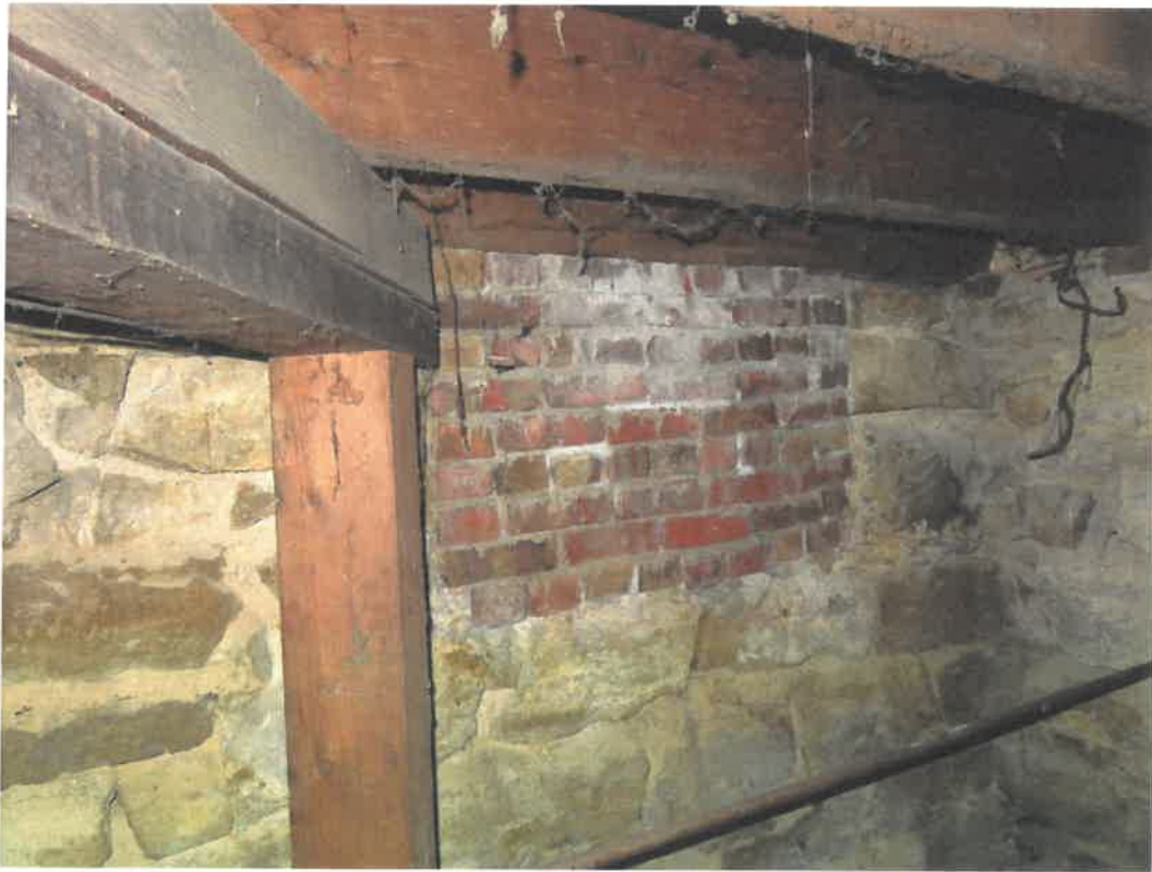
Photo 85 Building No. 36 – Hasselbach Pharmacy (143 S 3rd St) Brick Filled-In Coal Chute in Basement
