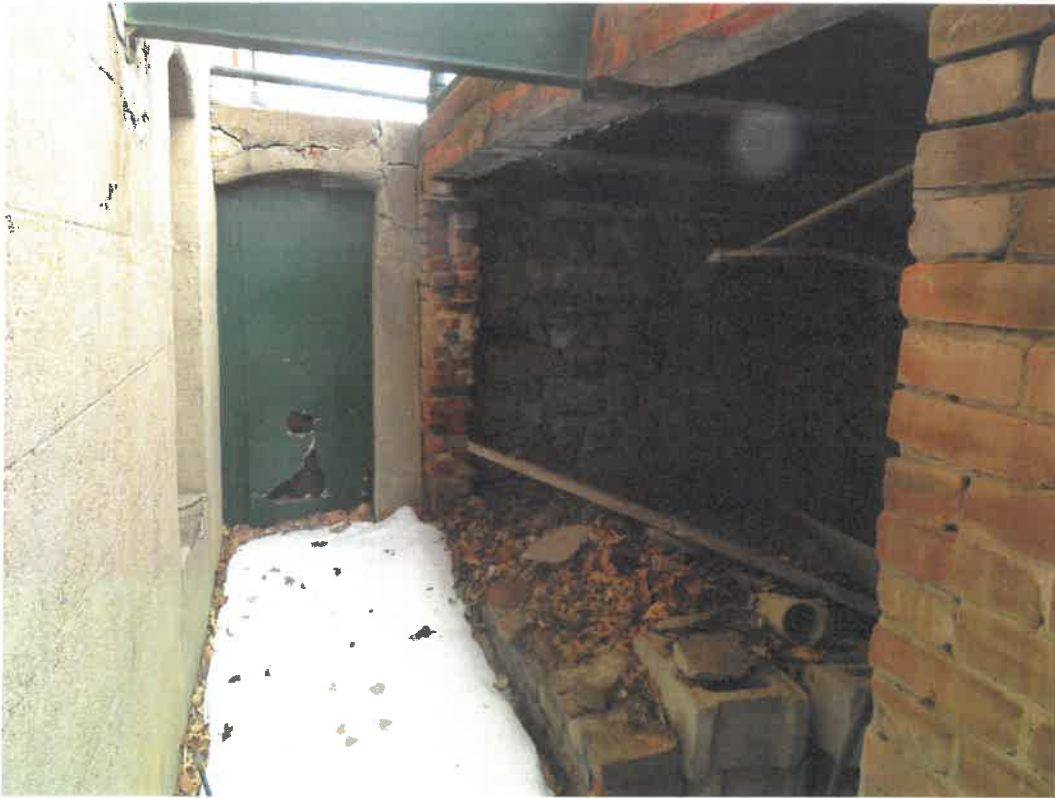
Photo 31 Building No. 17 – Nester & Mercure Attorneys (398 Broadway St) Fallen Wall at North End of Vault 1 w/ Vault 2 South Walk Door
