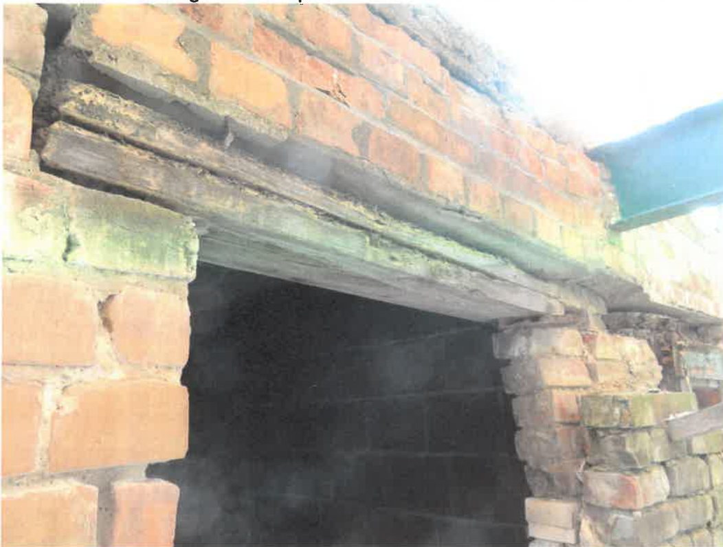
Photo 30 Building No. 17 – Nester & Mercure Attorneys (398 Broadway St) Typical Deterioration of Walk Door in Vault 1
