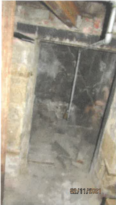
Photo 99 Building No. 41 – Col. Barney Oldfield Education Center (175 S 3rd St) Door Opening to Vault in Basement
