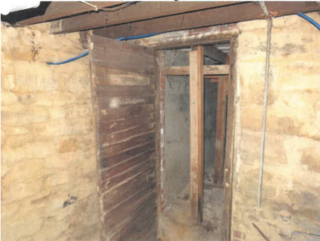
Photo 106 Building No. 43 – Farm Bureau Financial Services (185 S 3rd St) Open Door to Vault in Basement of Building
