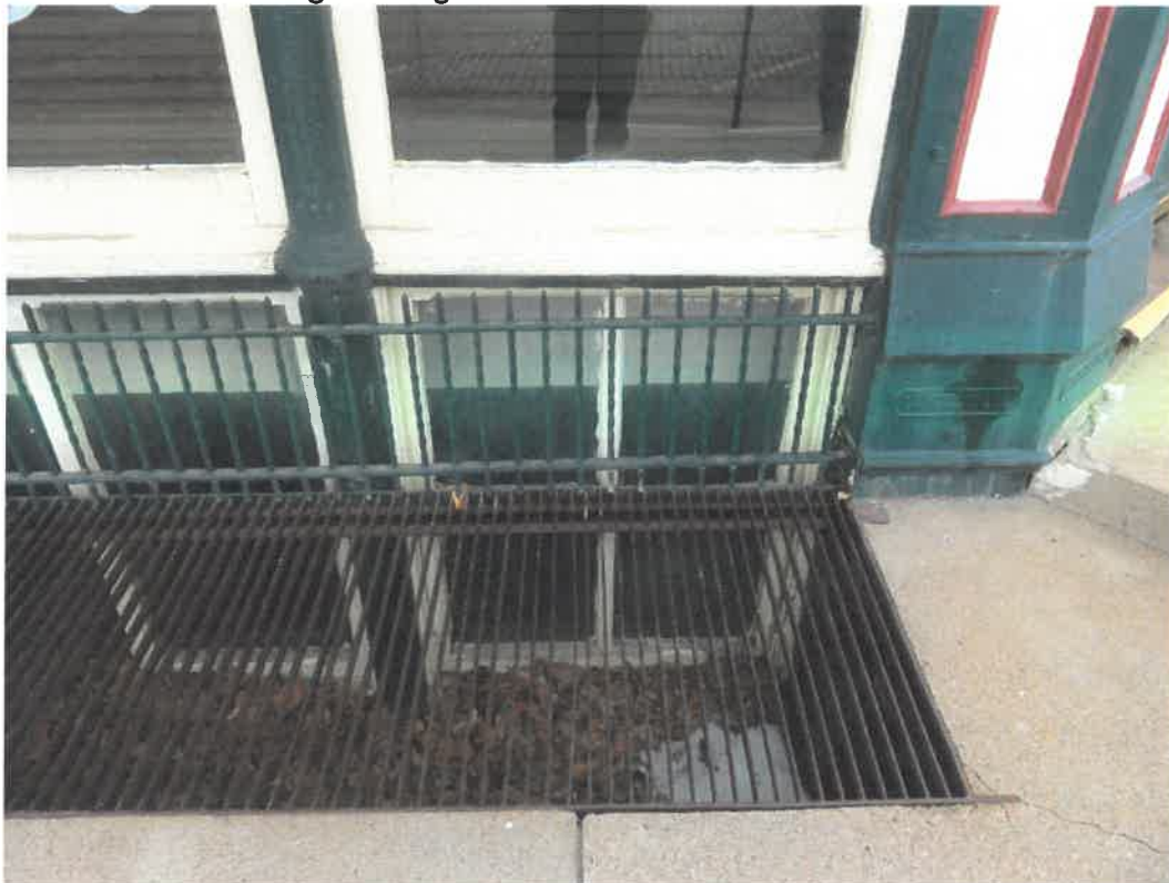
Photo 20 Building No. 17 – Nester & Mercure Attorneys (398 Broadway St) Lightwell on South Side of Frontage
