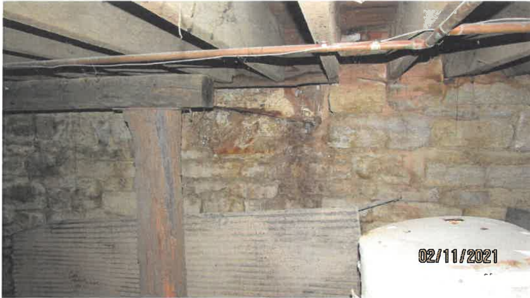
Photo 117 Building No. 45 – Hair by Luann (195 S 3rd St) Rubble Limestone Filled-In Coal Chute on South Face of Building in Basement
