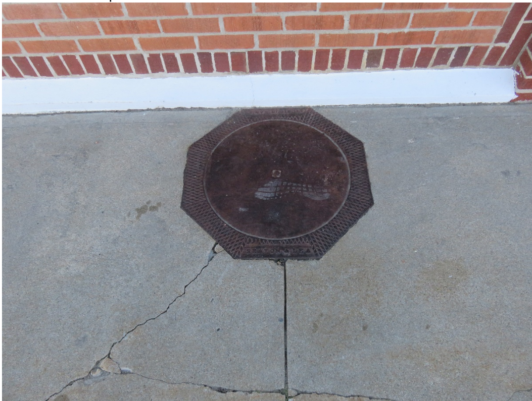
Photo 146 Building No. 56 – Brinkman’s Chevrolet & Buick (301/305/306 Clay St) Open Manhole in Sidewalk of East Annex
