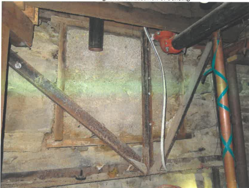
Photo 48 Building No. 22 – Hopkins Block (340 Broadway St) Concrete Filled-In Lightwell on East Half of Building
