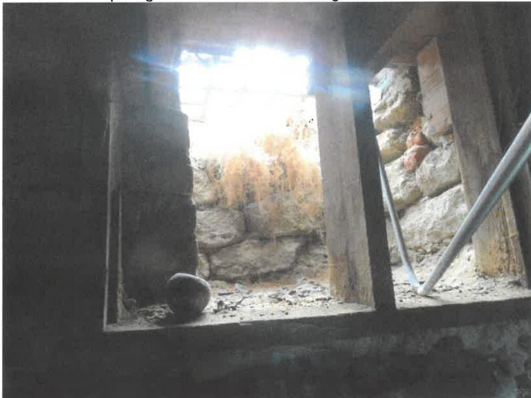
Photo 50 Building No. 22 – Hopkins Block (340 Broadway St) Open Lightwell on West Half of Building
