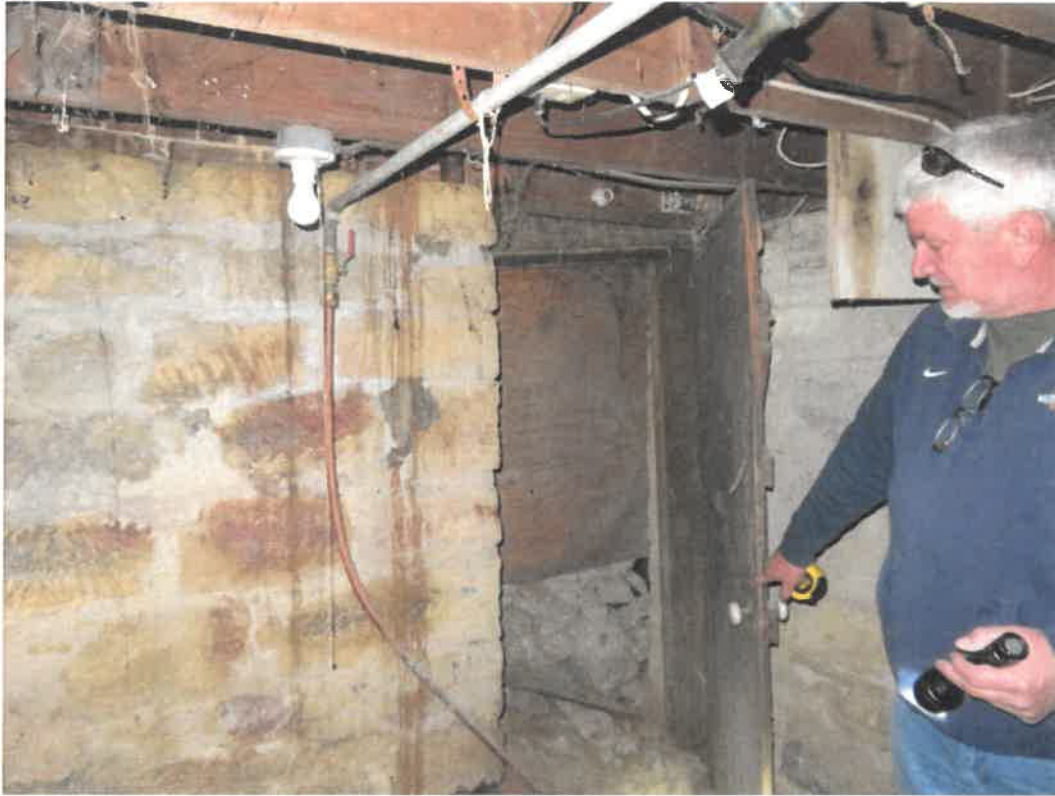
Photo 119 Building No. 46 – Blessing Heating & Plumbing (276 Clay St) Open Door in Basement to Vault Under Sidewalk
