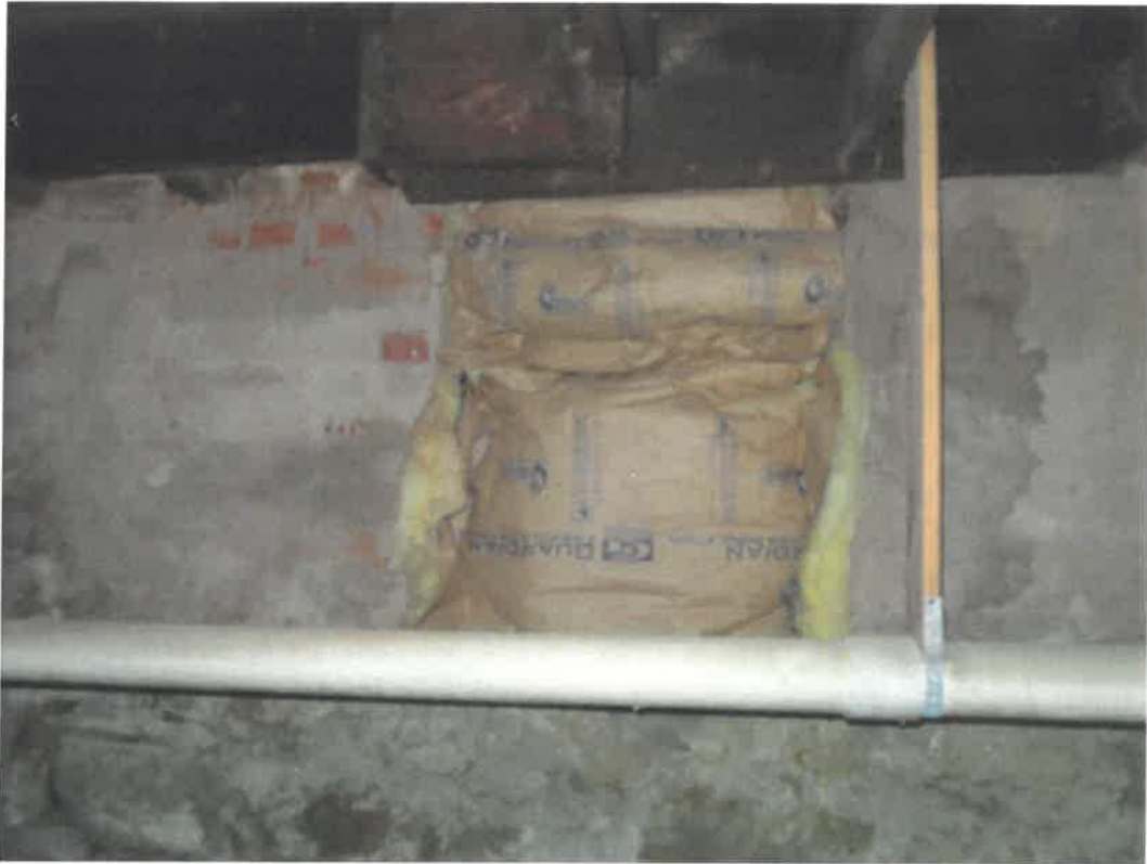
Photo 159 Building No. 59 – Tecumseh Central Market (381 Clay St) Partially Filled in Vent Opening in Basement on East Side of East Annex
