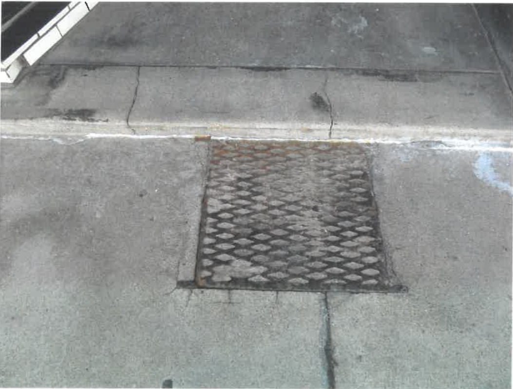
Photo 101 Building No. 42 – Morrissey, Morrissey & Dalluge (177 S 3rd St) Concrete Filled-In Coal Chute in Sidewalk
