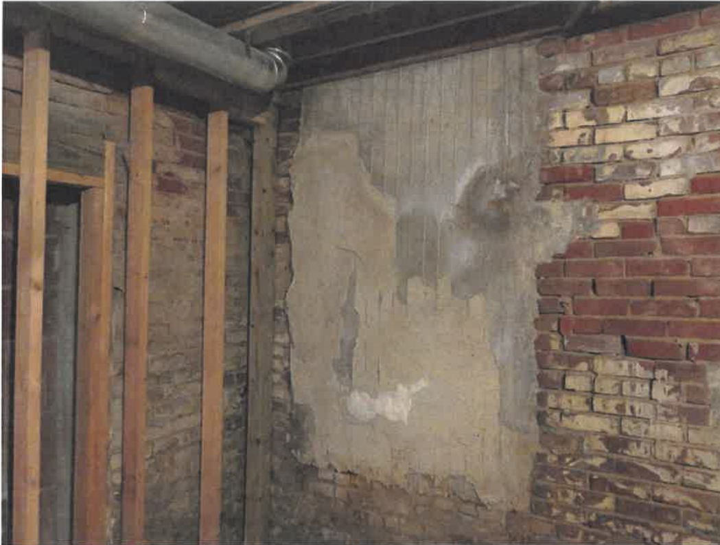
Photo 141 Building No. 55 – Johnson County Museum (235 S 3rd St) Concrete Filled-In Coal Chute on North Wall of Basement
