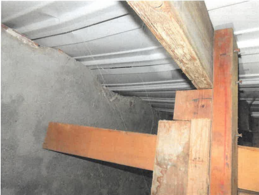
Photo 105 Building No. 43 – Farm Bureau Financial Services (185 S 3rd St) Metal Form Deck/Wood Framing/Concrete Wall of Vault Under Sidewalk
