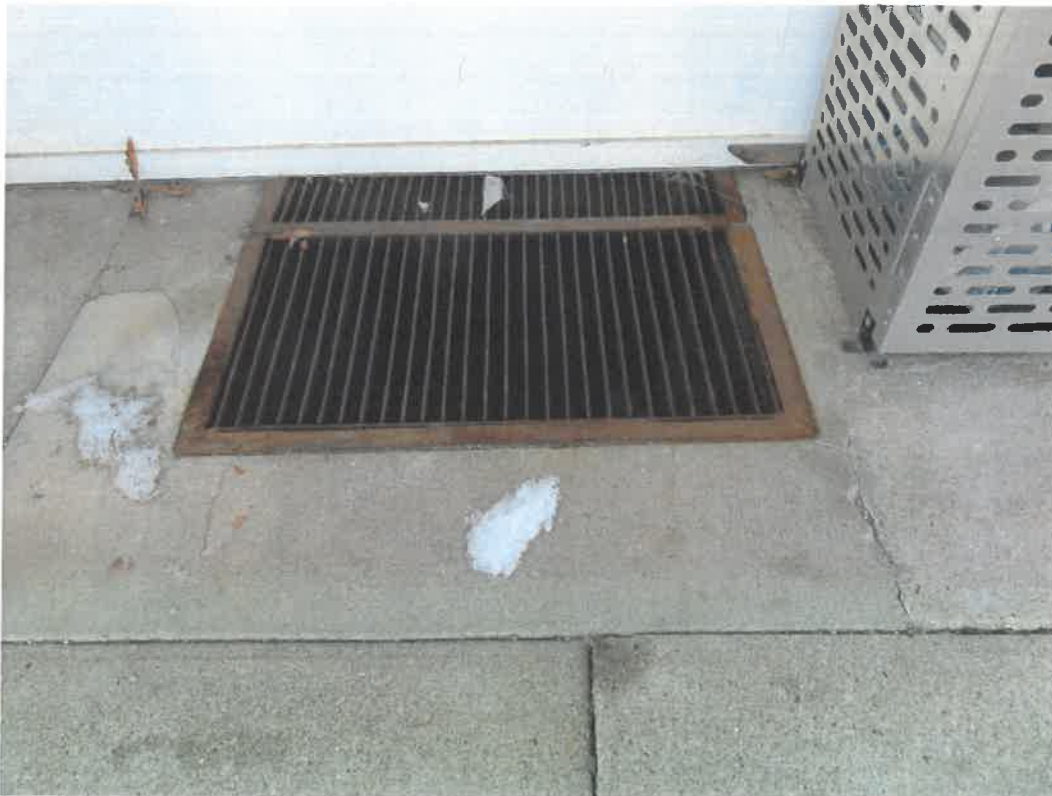
Photo 155 Building No. 59 – Tecumseh Central Market (381 Clay St) Open Vent in Sidewalk on North Side of Building
