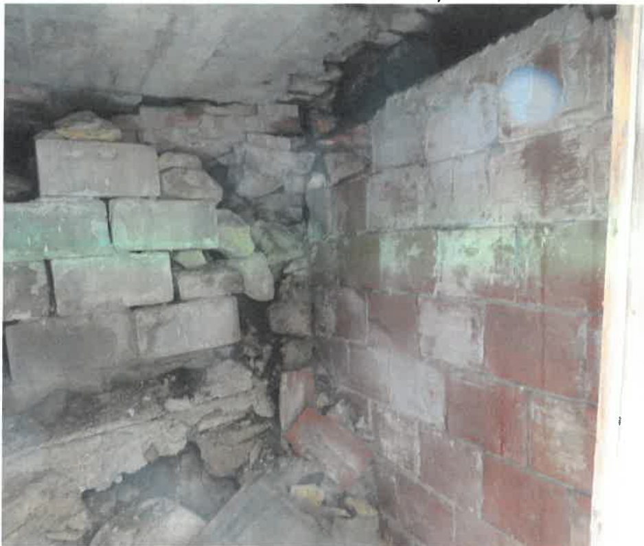
Photo 32 Building No. 17 – Nester & Mercure Attorneys (398 Broadway St) Typical Deterioration of Limestone & Hollow Clay Tile Foundation in Vault 1
