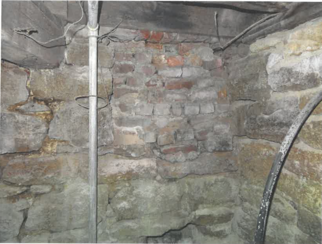
Photo 81 Building No. 35 – Chuck Ebeler Insurance & Investments (137 S 3rd St) Limestone/Brick Filled-In Coal Chute in Basement
