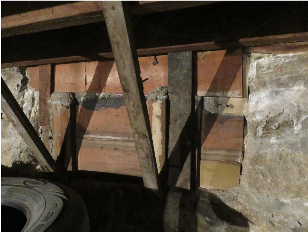
Photo 147 Building No. 56 – Brinkman’s Chevrolet & Buick (301/305/306 Clay St) Concrete Filled-In Coal Chute in Basement
