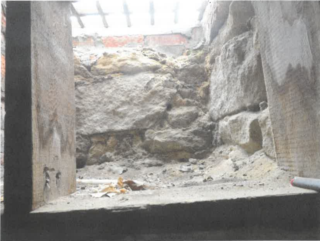
Photo 49 Building No. 22 – Hopkins Block (340 Broadway St) Open Lightwell on West Half of Building
