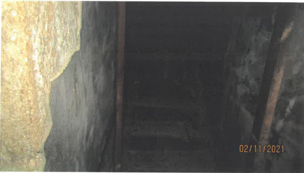
Photo 97 Building No. 41 – Col. Barney Oldfield Education Center (175 S 3rd St) Stair of Vault Under Sidewalk
