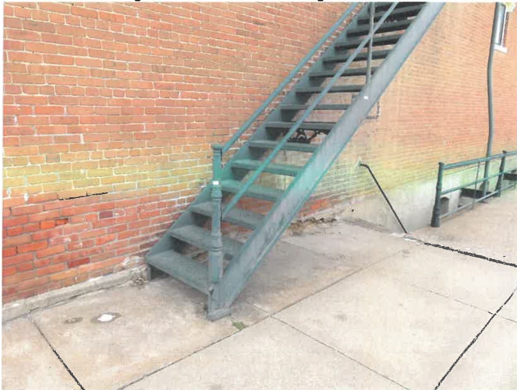
Photo 24 Building No. 17 – Nester & Mercure Attorneys (398 Broadway St) Stairs to 2 nd Floor & Stair/Hall to Basement on East Side of Building
