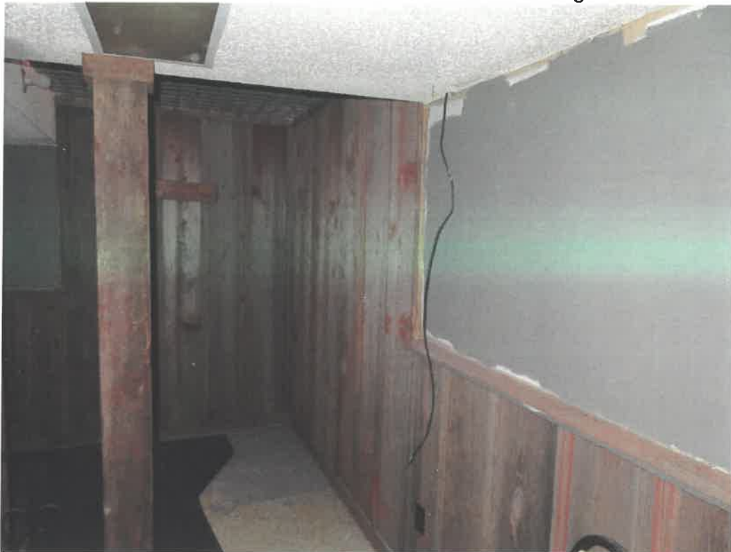
Photo 40 Building No. 20 – TNT Smoke House (366 Broadway St) Typical Finish Covering Up Coal Chute on East Half of Building
