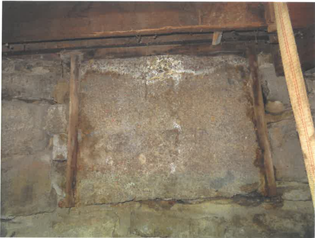
Photo 47 Building No. 22 – Hopkins Block (340 Broadway St) Concrete Filled-In Lightwell on East Half of Building
