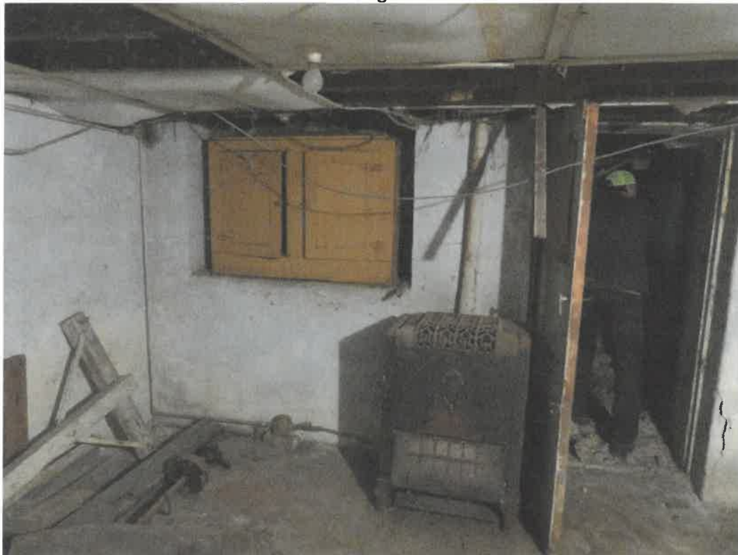
Photo 124 Building No. 47 – Hupka Farm Toys (266 Clay St) Open Door & Window in Basement to Vault Under Sidewalk
