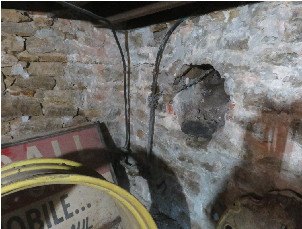
Photo 148 Building No. 56 – Brinkman’s Chevrolet & Buick (301/305/306 Clay St) Open Manhole Opening in Basement
