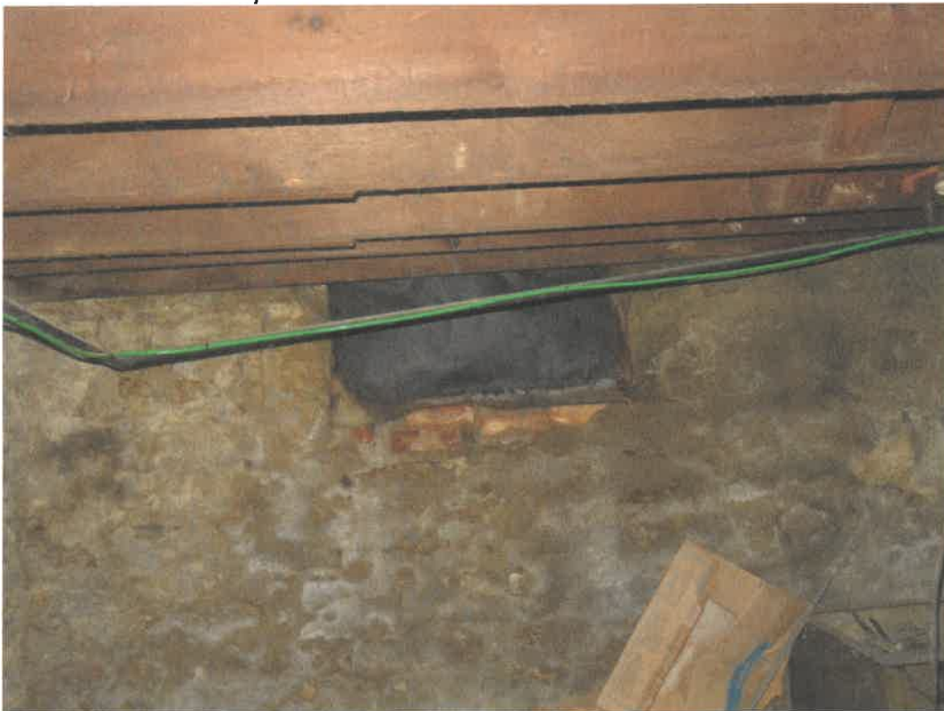
Photo 56 Building No. 24 – Broadway Beauty & Bargains (318 Broadway St) Partially Filled-In Coal Chute Using Fabric in Basement
