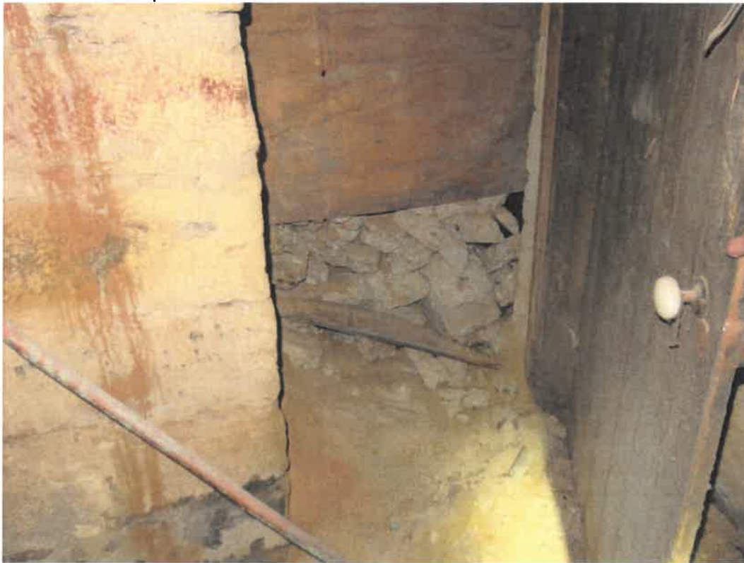
Photo 120 Building No. 46 – Blessing Heating & Plumbing (276 Clay St) Open Door in Basement to Vault Under Sidewalk
