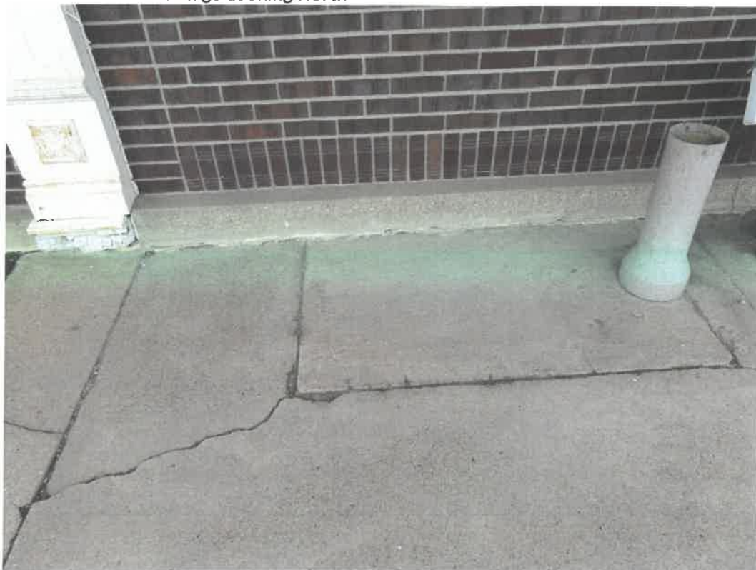
Photo 38 Building No. 20 – TNT Smoke House (366 Broadway St) Concrete Filled-In Coal Chute on East Half of Building
