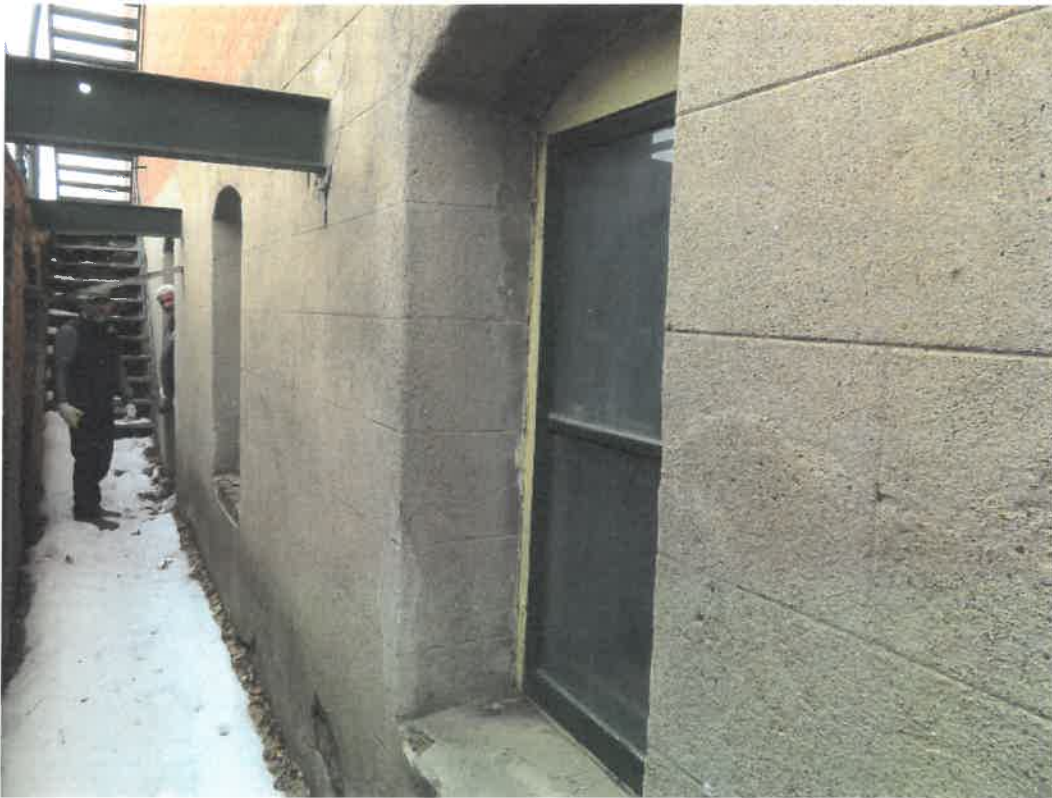
Photo 27 Building No. 17 – Nester & Mercure Attorneys (398 Broadway St) Typical Windows in Basement Hall w/ Walk Door in the Distance
