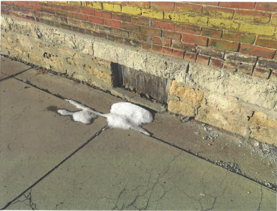
Photo 157 Building No. 59 – Tecumseh Central Market (381 Clay St) Typical Window Opening in Basement Wall on East Side of East Annex
