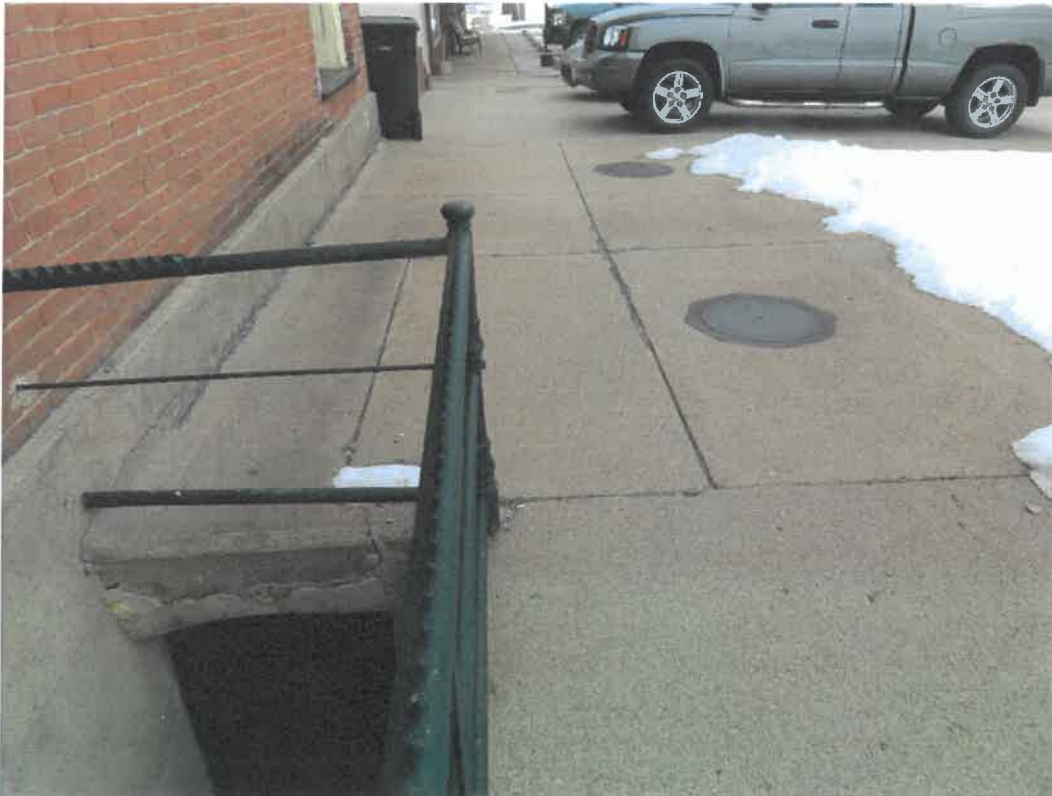
Photo 33 Building No. 17 – Nester & Mercure Attorneys (398 Broadway St) Looking North at Top of Vault 2 Under Sidewalk that Extends to Street Curb
