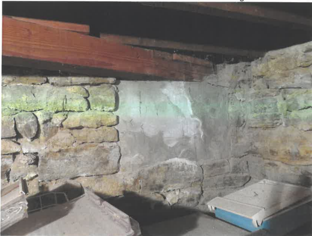
Photo 44 Building No. 21 – D.A. Wolken & Sons (362 Broadway St) Concrete Filled-In Coal Chute on West End of Building
