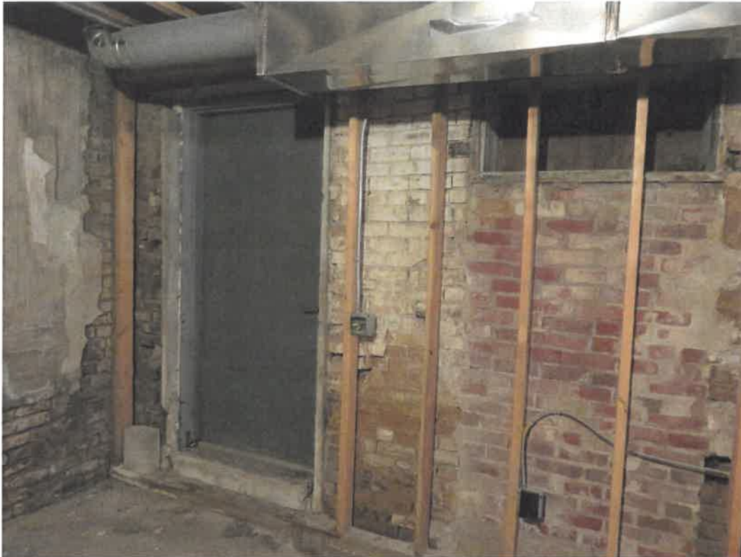
Photo 139 Building No. 55 – Johnson County Museum (235 S 3rd St) Open Door & Window to Exterior Stairway in Basement on East Side of Building
