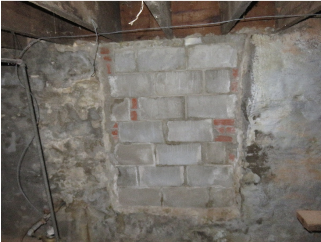
Photo 63 Building No. 26 – American National Bank (306/310 Broadway St) CMU/Brick Filled-In Window at South End of West Wall in Basement
