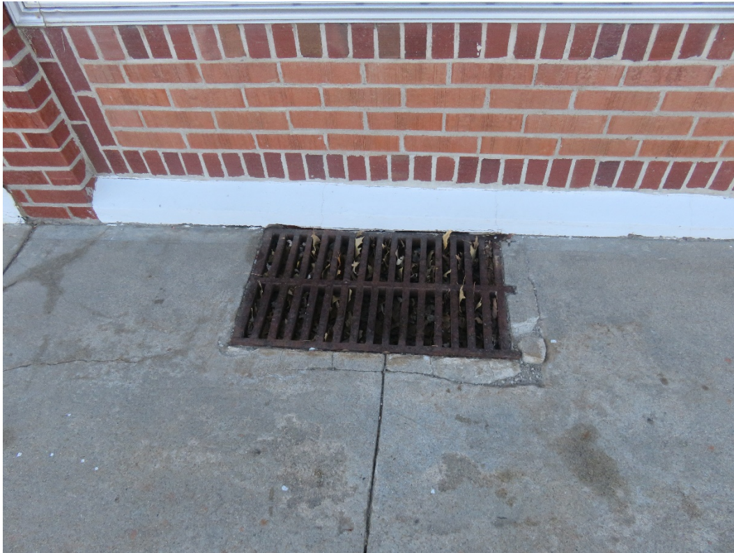
Photo 145 Building No. 56 – Brinkman’s Chevrolet & Buick (301/305/306 Clay St) Open Coal Chute in Sidewalk of East Annex
