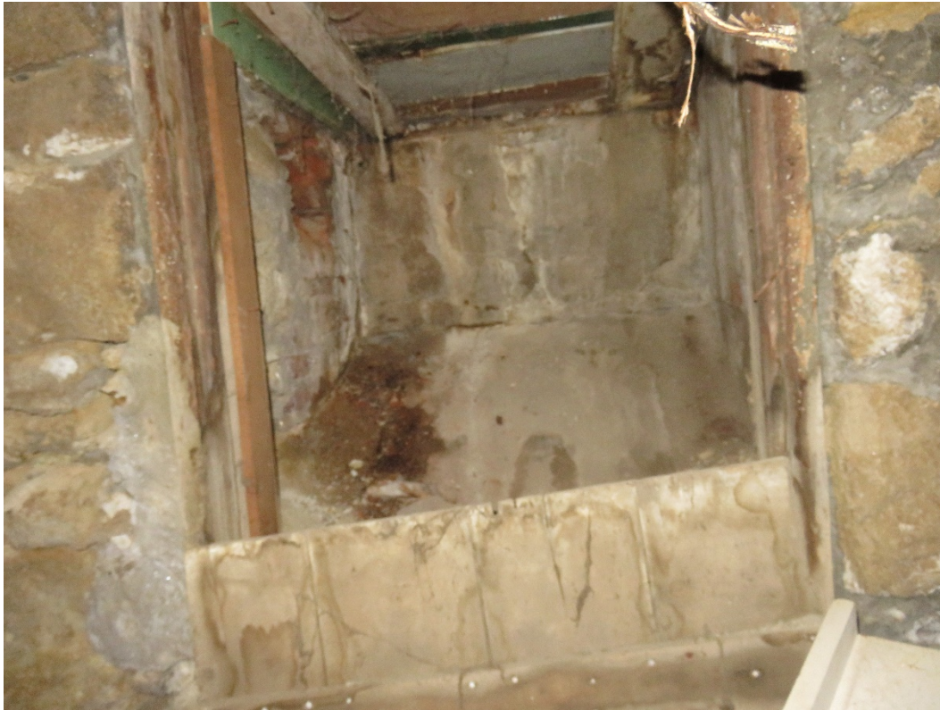
Photo 75 Building No. 33 – Tecumseh Chieftain (117 S 3rd St) Open Coal Chute in Basement
