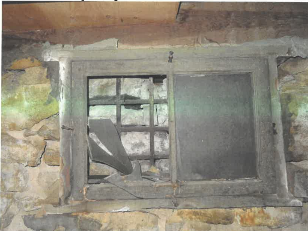
Photo 58 Building No. 25 – American National Bank – East Annex (310 Broadway St) Rubble Limestone Filled-In Window in Basement
