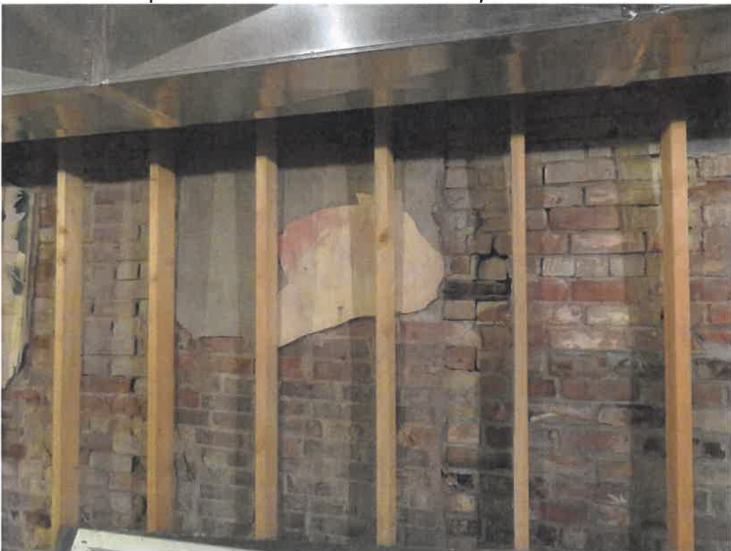
Photo 140 Building No. 55 – Johnson County Museum (235 S 3rd St) Concrete Filled-In Coal Chute on North Wall of Basement
