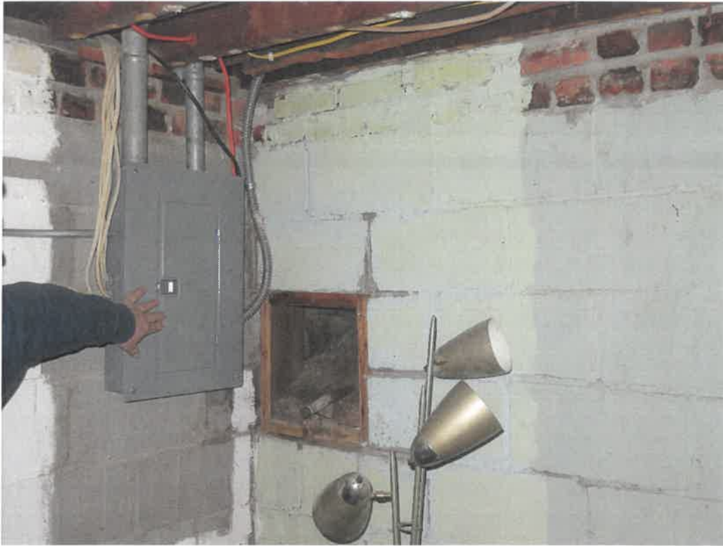
Photo 109 Building No. 44 – To Gather On the Square (193 S 3rd St) Opening for Water Shut-off in Basement of Building
