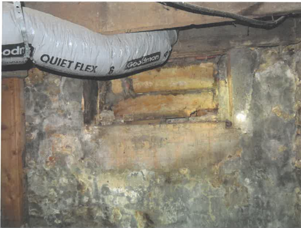
Photo 151 Building No. 57 – Darel Weber Real Estate (335 Clay St) Rubble Filled-In Coal Chute in Basement
