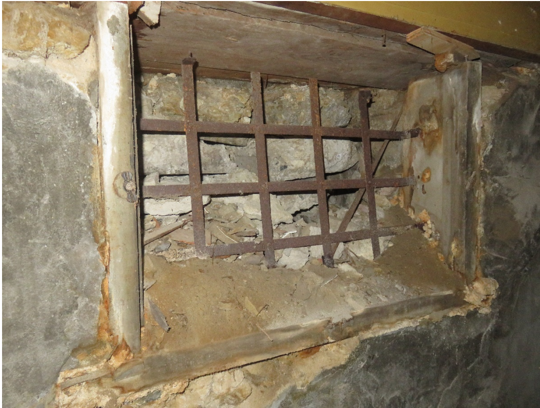
Photo 59 Building No. 25 – American National Bank – East Annex (310 Broadway St) Rubble Limestone Filled-In Window in Basement
