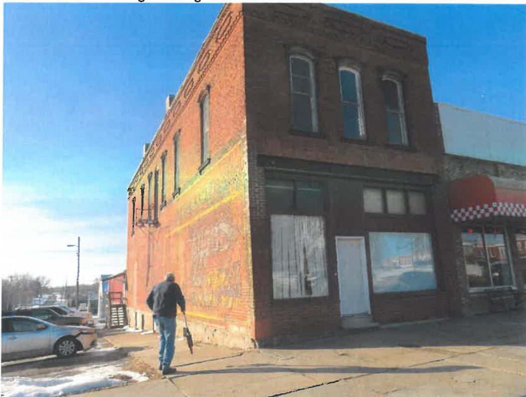
Photo 154 Building No. 59 – Tecumseh Central Market – East Annex (381 Clay St) East Annex Frontage Looking Southwest
