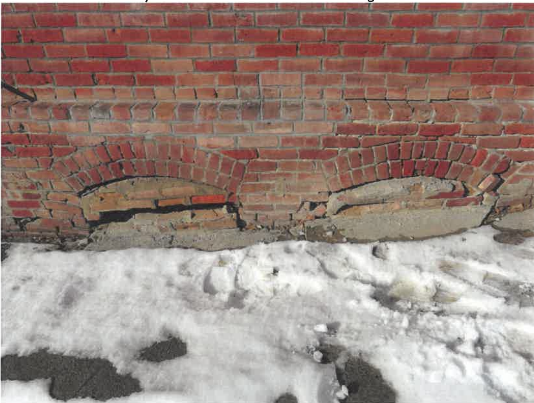
Photo 138 Building No. 55 – Johnson County Museum (235 S 3rd St) Arched Windows of Basement Exposed Above Sidewalk on East Side of Building
