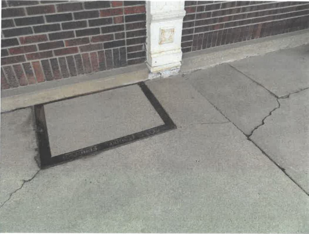
Photo 39 Building No. 20 – TNT Smoke House (366 Broadway St) Concrete Filled-In Coal Chute on West Half of Building
