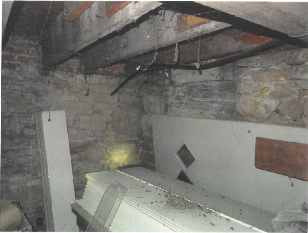
Photo 77 Building No. 34 – Chief Rexall Drugs (123 S 3rd St) Limestone Filled-In Coal Chute in Basement
