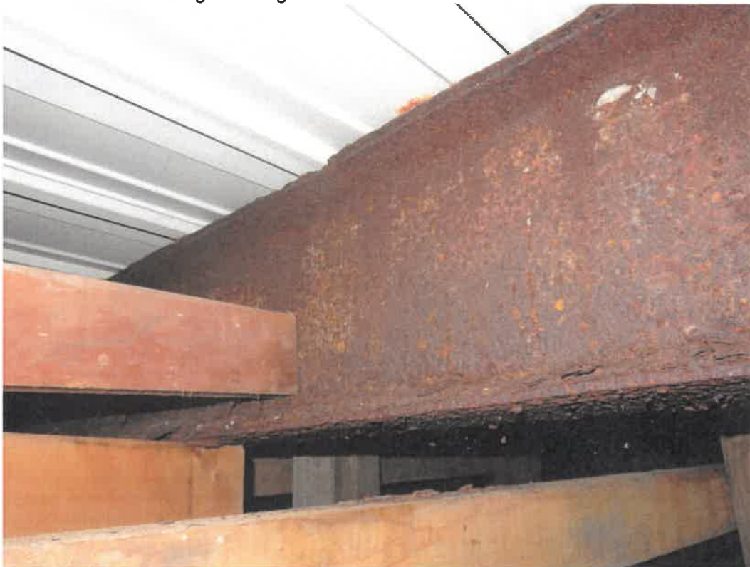
Photo 104 Building No. 43 – Farm Bureau Financial Services (185 S 3rd St) Steel Beam/Metal Form Deck/Wood Framing of Vault Under Sidewalk
