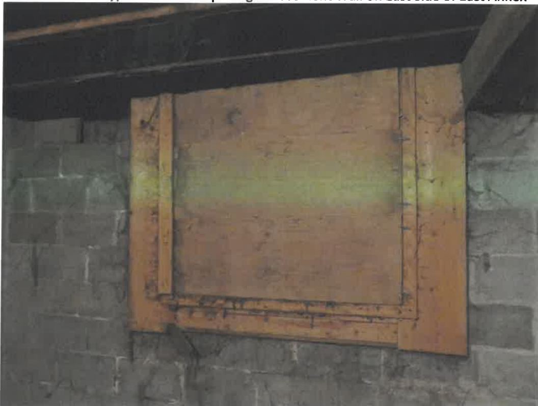
Photo 158 Building No. 59 – Tecumseh Central Market – East Annex (381 Clay St) Vent Opening in Basement Wall on North Side of Building
