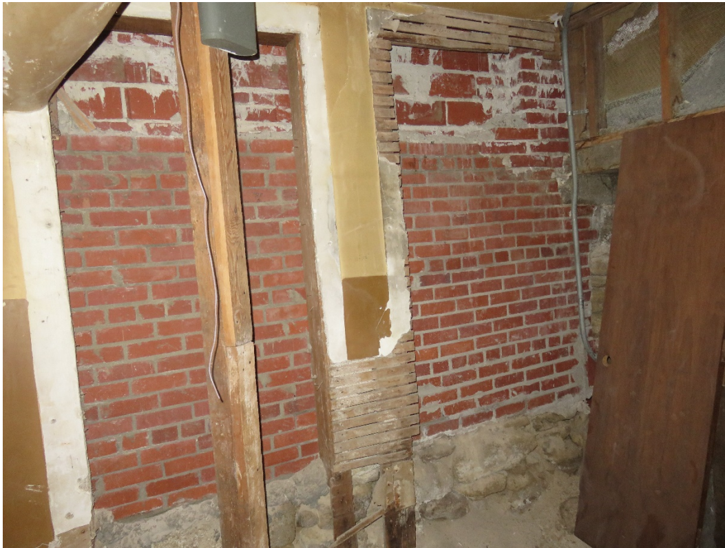
Photo 62 Building No. 26 – American National Bank (306/310 Broadway St) Brick Filled-In Vault at West End of South Wall in Basement
