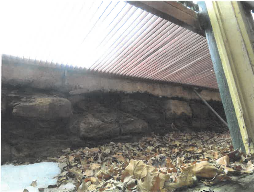
Photo 23 Building No. 17 – Nester & Mercure Attorneys (398 Broadway St) Grating & Limestone Foundation of Lightwell
