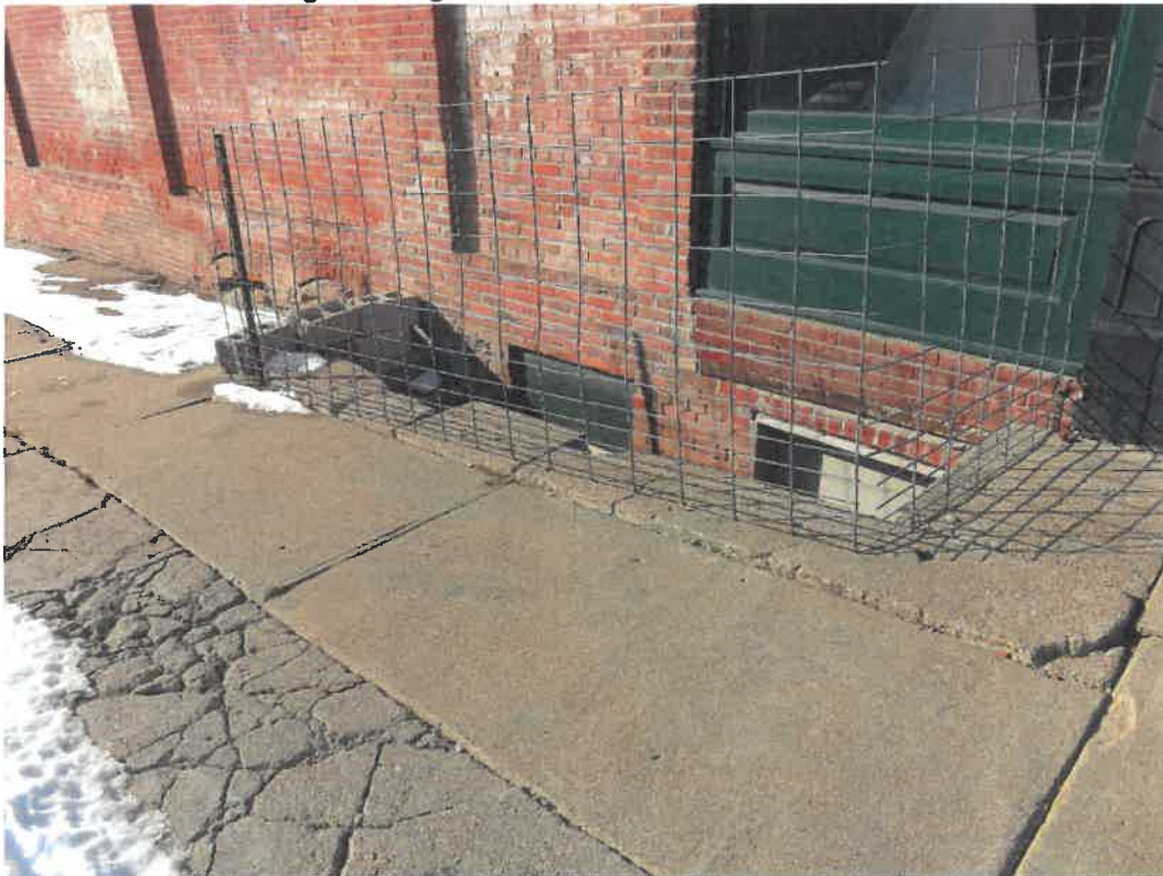
Photo 136 Building No. 55 – Johnson County Museum (235 S 3rd St) Open Stairway in Sidewalk on East Face of Building
