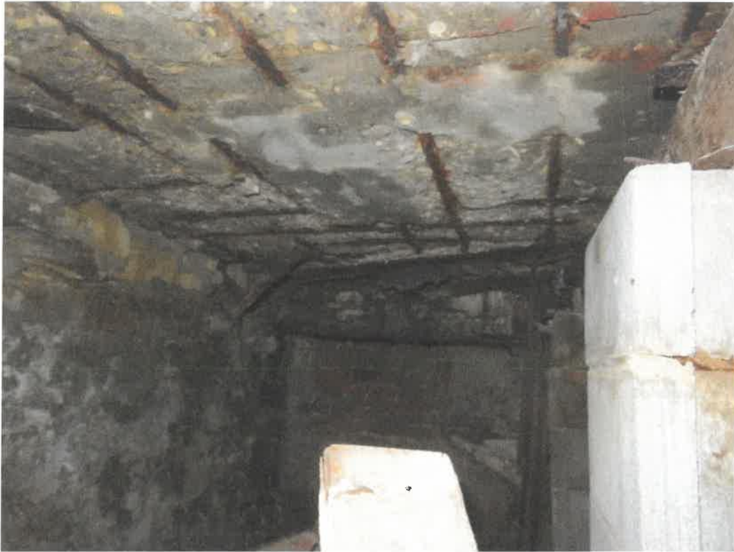
Photo 123 Building No. 47 – Hupka Farm Toys (266 Clay St) Vault Under Sidewalk Looking West
