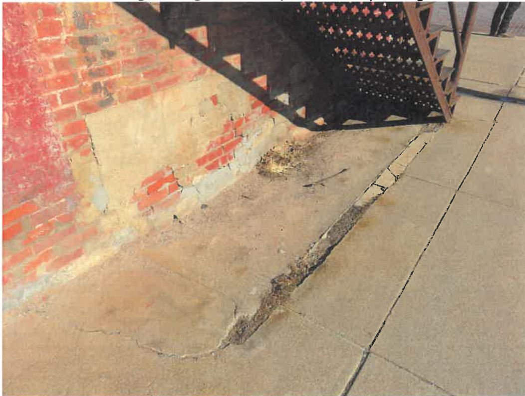
Photo 112 Building No. 45 – Hair by Luann (195 S 3rd St) Concrete Filled-In Stairway in Sidewalk on South Face of Building
