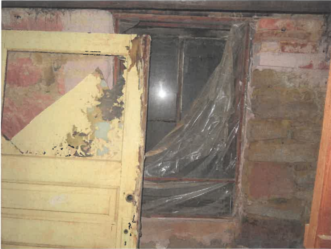
Photo 107 Building No. 43 – Farm Bureau Financial Services (185 S 3rd St) Open Window to Vault in Basement of Building
