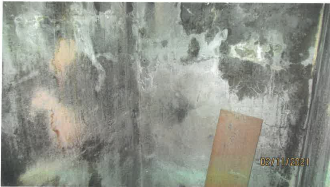
Photo 98 Building No. 41 – Col. Barney Oldfield Education Center (175 S 3rd St) Vault Under Sidewalk
