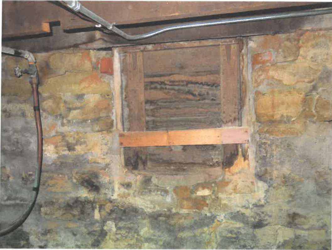
Photo 91 Building No. 38 – Ramsey Family Fountain (155 S 3rd St) Wood Plank Filled-In Coal Chute in Basement
