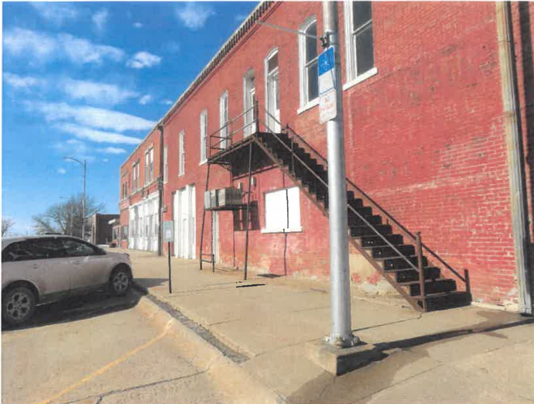
Photo 111 Building No. 45 – Hair by Luann (195 S 3rd St) Frontage Looking Northwest w/ Steel Stairway Leading to 2 nd Floor
