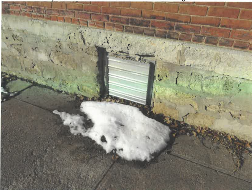
Photo 156 Building No. 59 – Tecumseh Central Market – East Annex (381 Clay St) Vent Opening in Basement Wall on East Side of East Annex
