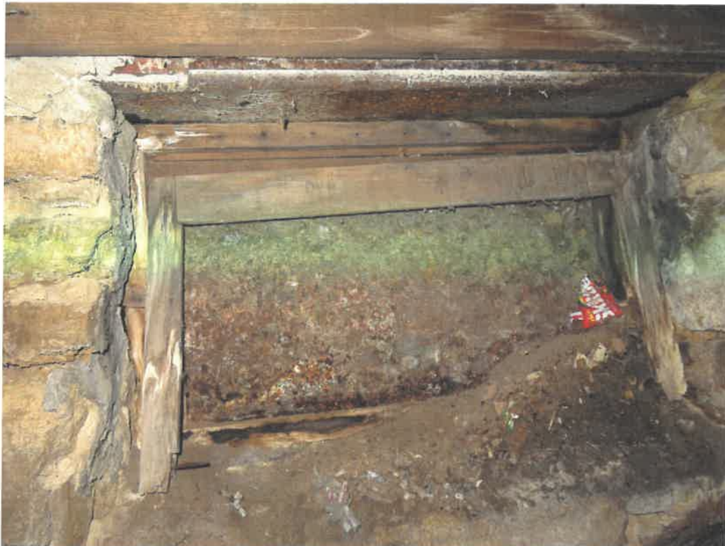
Photo 84 Building No. 36 – Hasselbach Pharmacy (143 S 3rd St) Soil Filled-In Window in Basement
