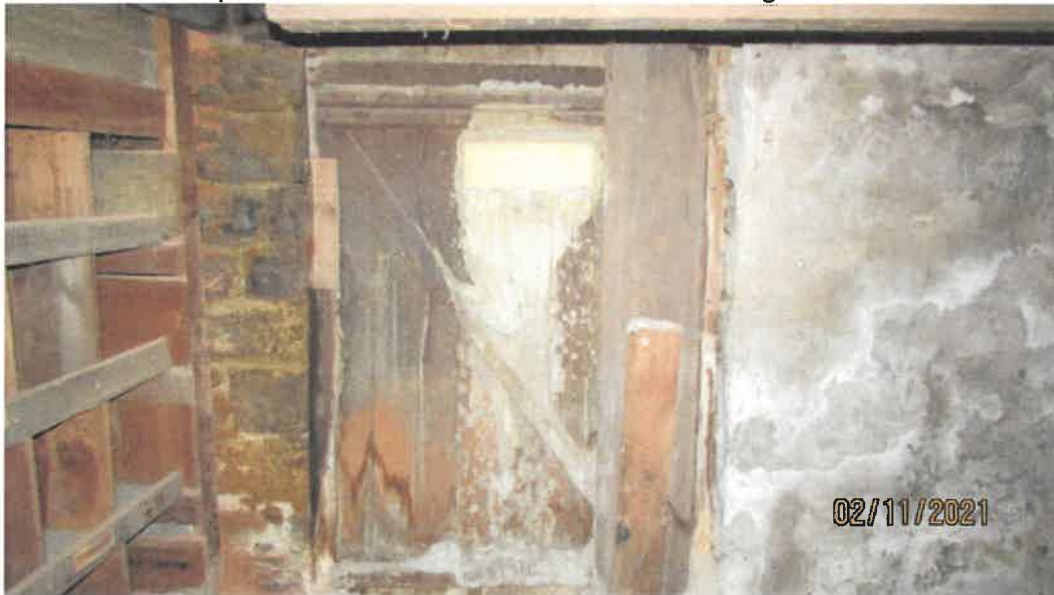
Photo 114 Building No. 45 – Hair by Luann (195 S 3rd St) Concrete Filled-In Door to Previous Stairway on South Face of Building
