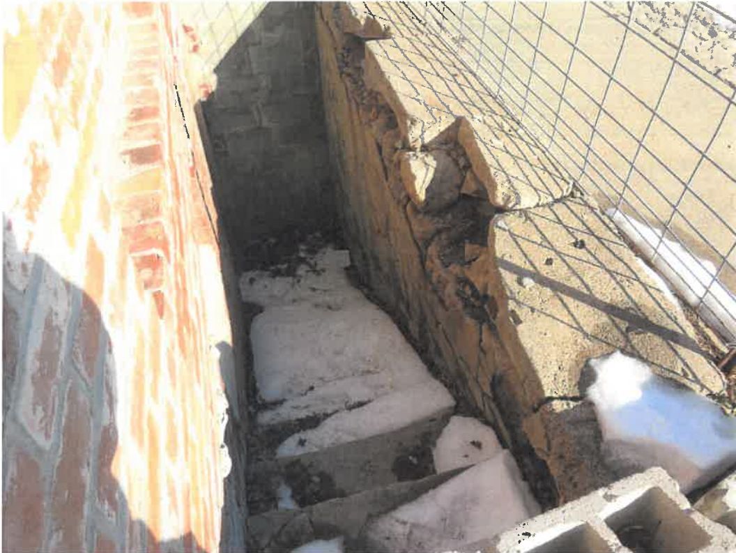
Photo 137 Building No. 55 – Johnson County Museum (235 S 3rd St) Stairway to Basement on East Side of Building
