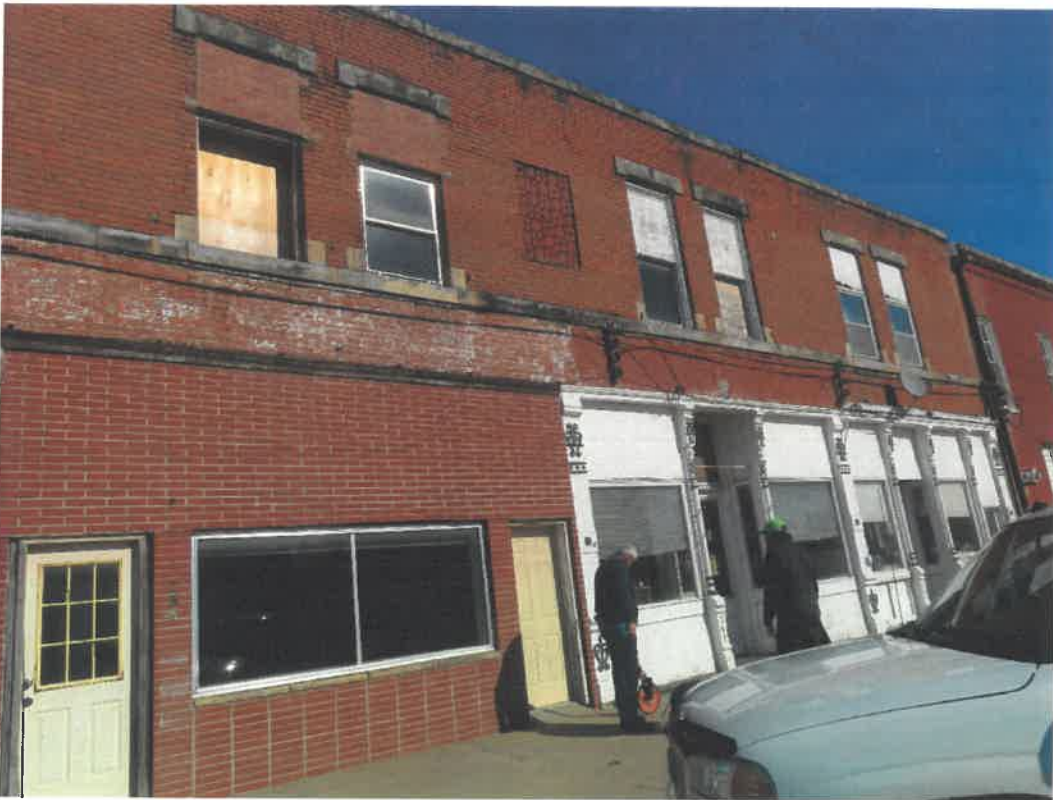
Photo 125 Building No. 48 – Tecumseh EDC Building (256 Clay St) Frontage Looking Northeast (Note: Vault Discovered Under Sidewalk)
