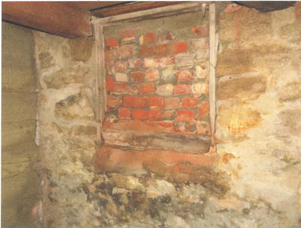
Photo 90 Building No. 38 – Ramsey Family Fountain (155 S 3rd St) Brick Filled-In Coal Chute in Basement
