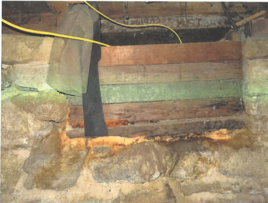
Photo 78 Building No. 34 – Chief Rexall Drugs (123 S 3rd St) Wood Plank Filled-In Coal Chute in Basement
