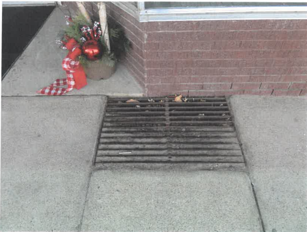
Photo 83 Building No. 36 – Hasselbach Pharmacy (143 S 3rd St) Soil Filled-In Coal Chute in Sidewalk
