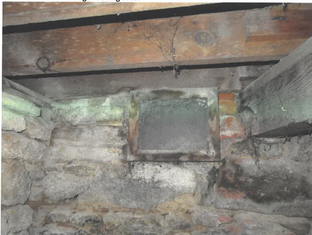
Photo 80 Building No. 35 – Chuck Ebeler Insurance & Investments (137 S 3rd St) Partially Filled-In Coal Chute Using Fabric in Basement
