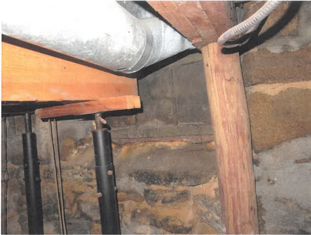
Photo 95 Building No. 40 – Flanigan’s On the Square (173 S 3rd St) Rubble Filled-In Coal Chute in Basement
