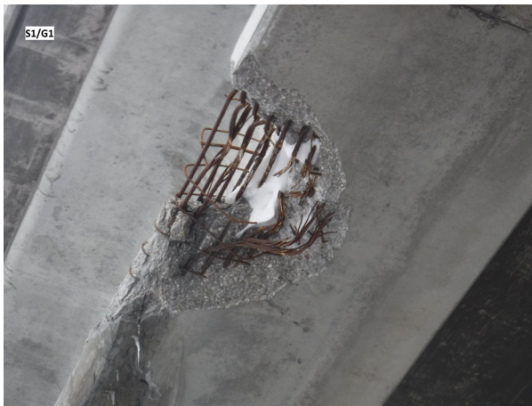
A. Strand Impact Damage
