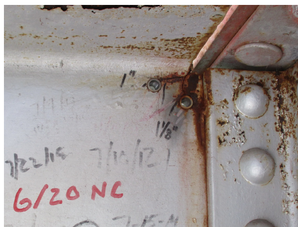
Figure 7.39—Crack Arresting Bushings on S012 00398
