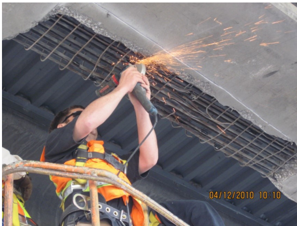
C. Cutting Damaged Strands
