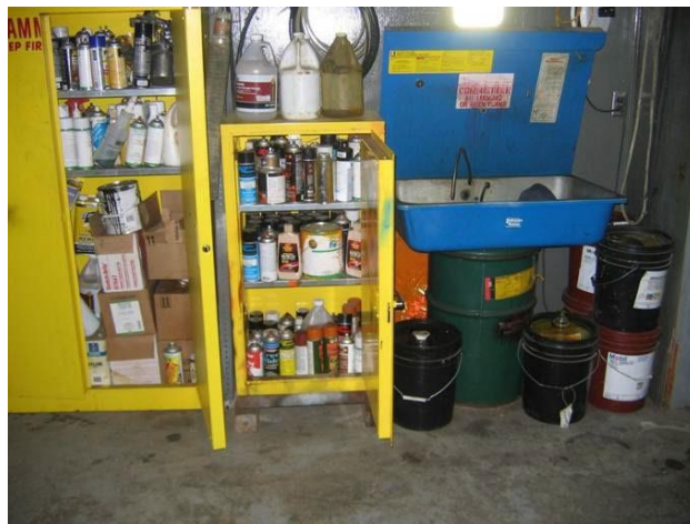
Multiple aerosols, paint cans, 5-gallon buckets, and a parts washer with 30-gallon drum.
