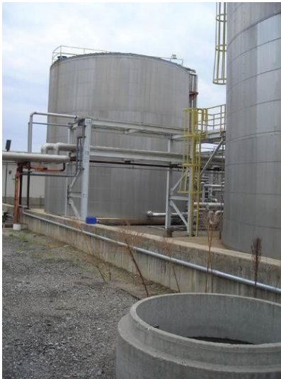
ASTs at a manufacturing plant.
