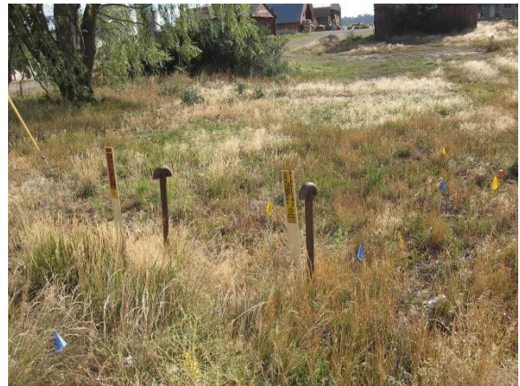
Gas pipeline vent pipes adjacent to highway right-of-way.
