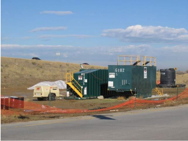
Baker remediation tank in highway right-of-way.
