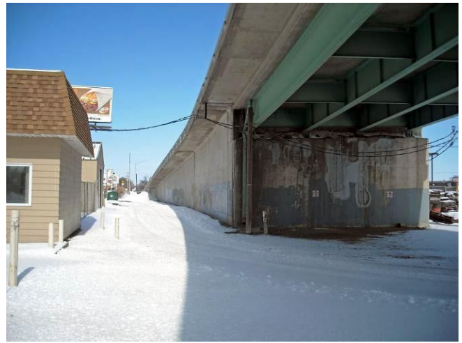
Paint on old bridges may contain heavy metal-based paint.
