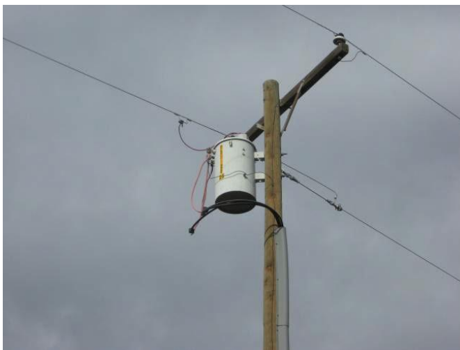
Pole-mounted electrical transformer in highway right-of-way.
