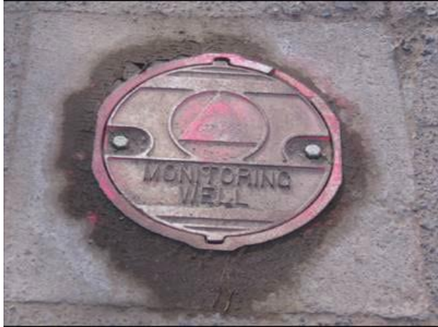
Flush mount monitoring well.
