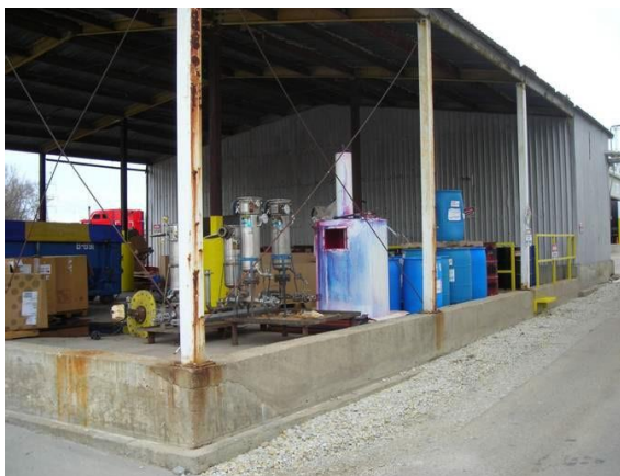
Covered hazardous materials storage area with secondary containment.
