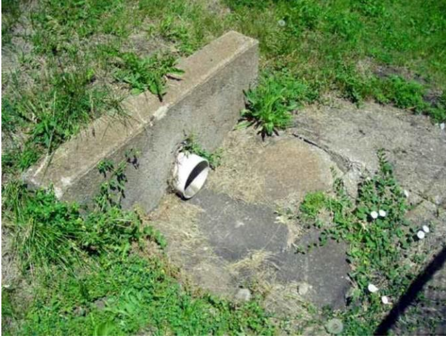
Drainpipe observed on the property of a foundry facility.
