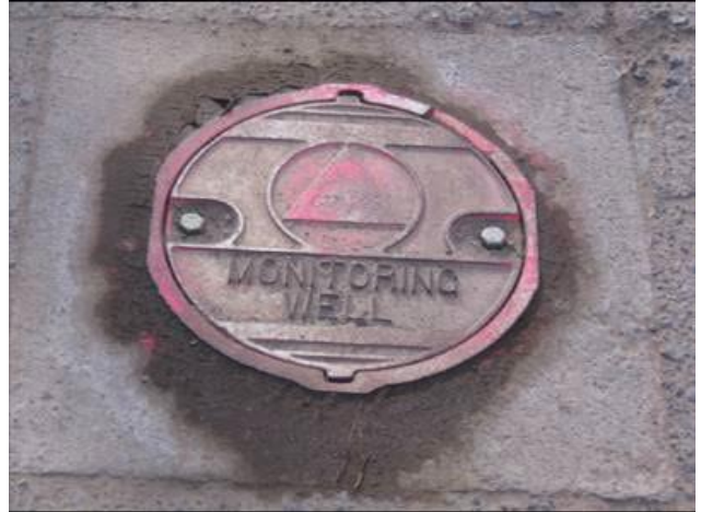
Typical in-ground monitoring well.
