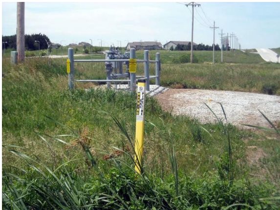
Gas line marker and regulator (background).
