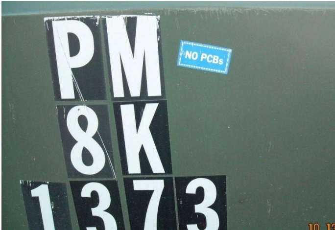
Pad-mounted electrical transformer.
