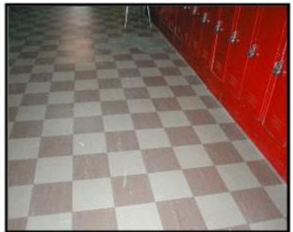
9 x 9 floor tiles commonly assumed to be ACM if made prior to 1980.
