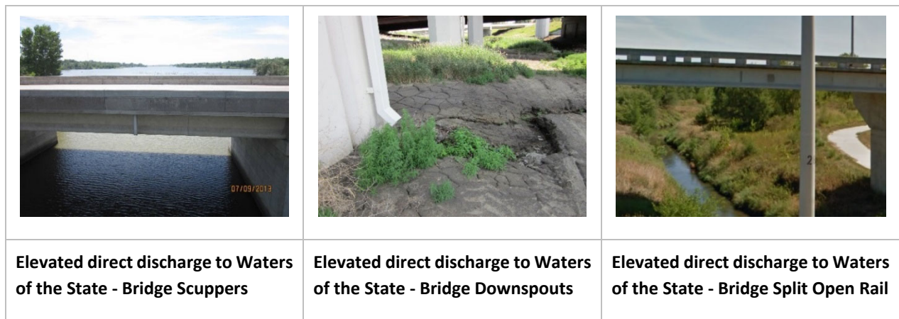
FIGURE 8. EXAMPLES OF ELEVATED MS4 OUTFALL DISCHARGES TO WATERS OF THE STATE
