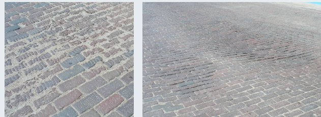
Significant deterioration Horizontal/vertical displacement
