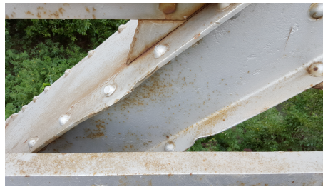
Fig. 27. Deformations of truss element
